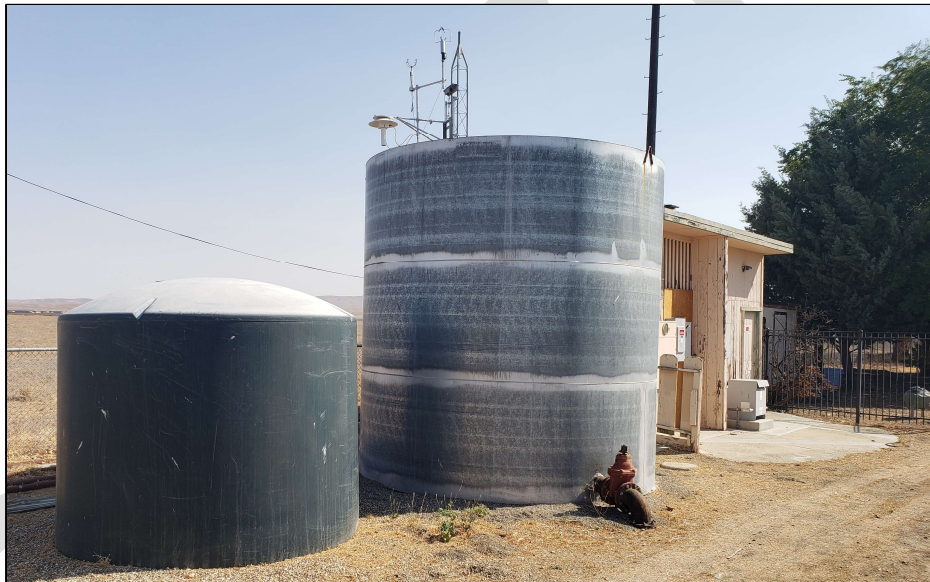
Figure 2-2. Left: Existing 2,500-gallon plastic tank (potable). Right: 10,000-gallon welded steel tank (irrigation).
