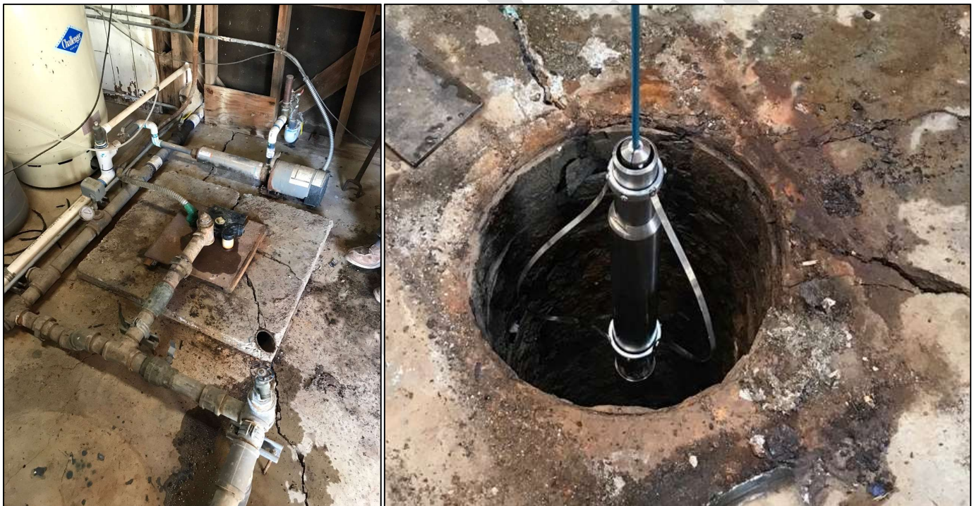
Figure 3-1. Left: Wellhead and one booster pump. Right: Inspection camera entering the heavily corroded well casing.
