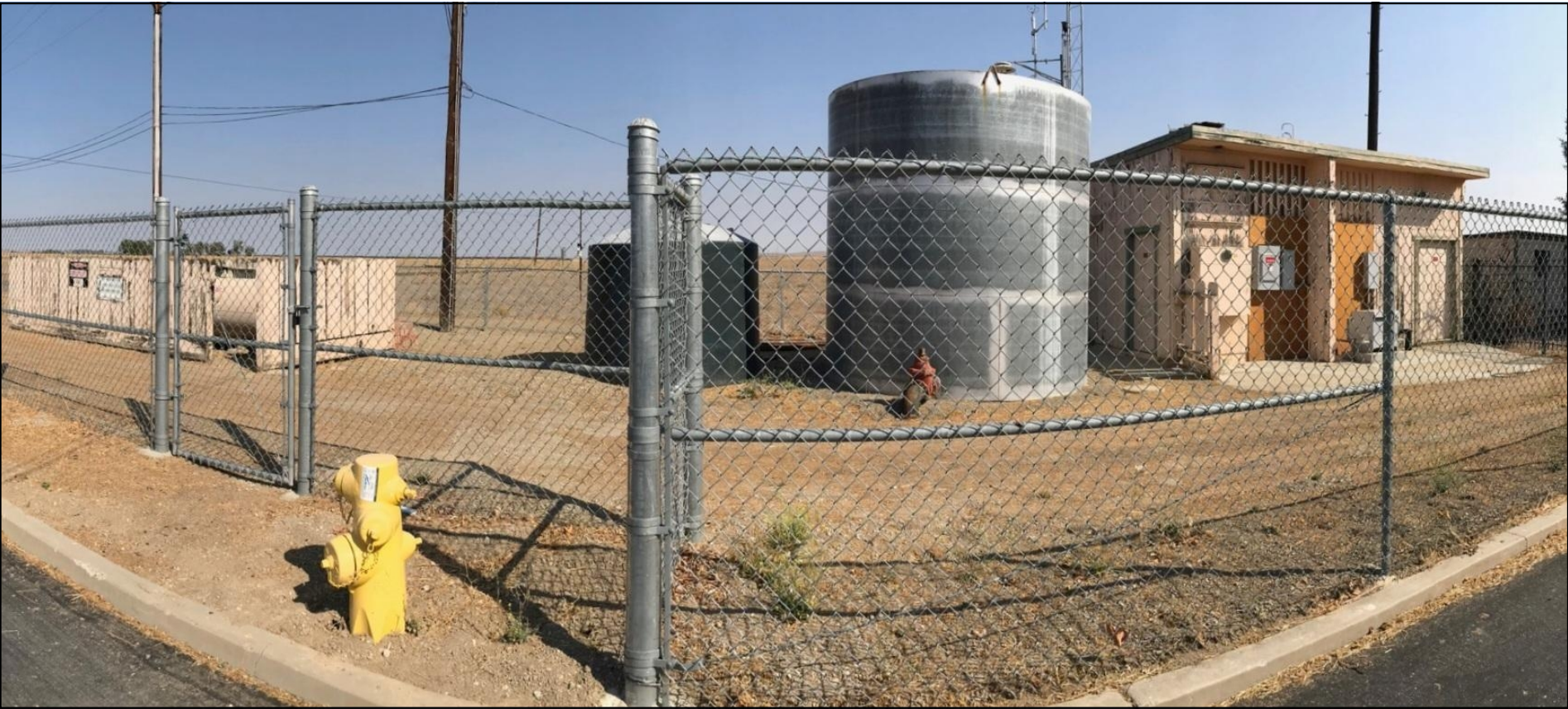
PHOTOGRAPH OF EXISTING CARRISA PLAINS ELEMENTARY WATER FACILITIES
