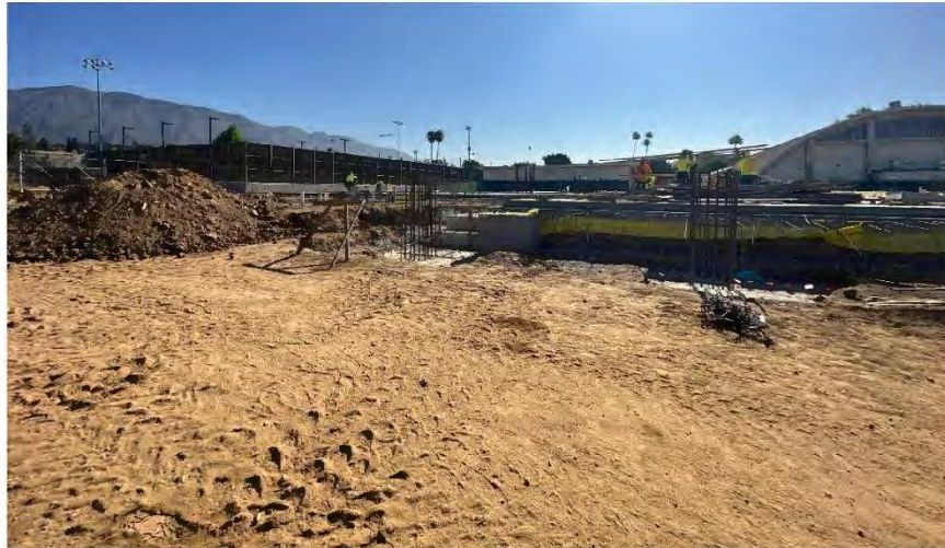
Facing west towards the Project site, at the location of the former tennis courts that is now developed with the building foundation.
