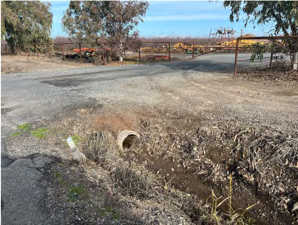
Photograph 29: From the eastern shoulder of Escalon-Bellota Road, looking northeast at an existing culvert located at 14159 County Highway Junction-6.
