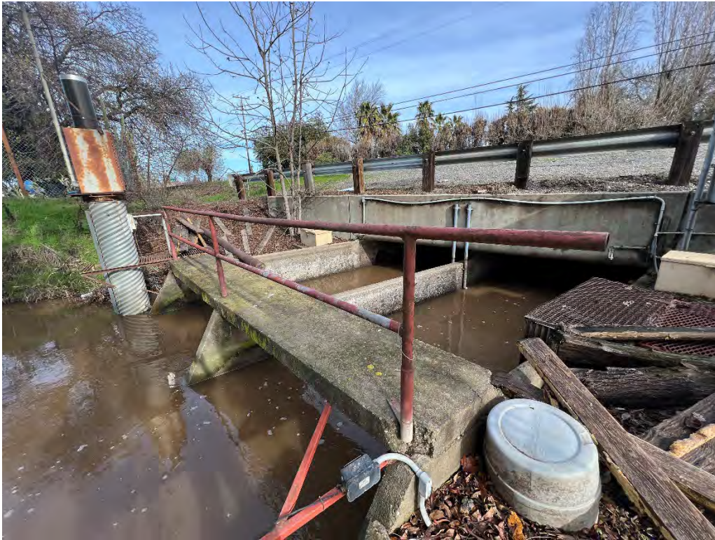
Photograph 21: From the southern bank of Lone Tree Creek, looking northeast through existing supporting structures toward Escalon-Bellota Road.
