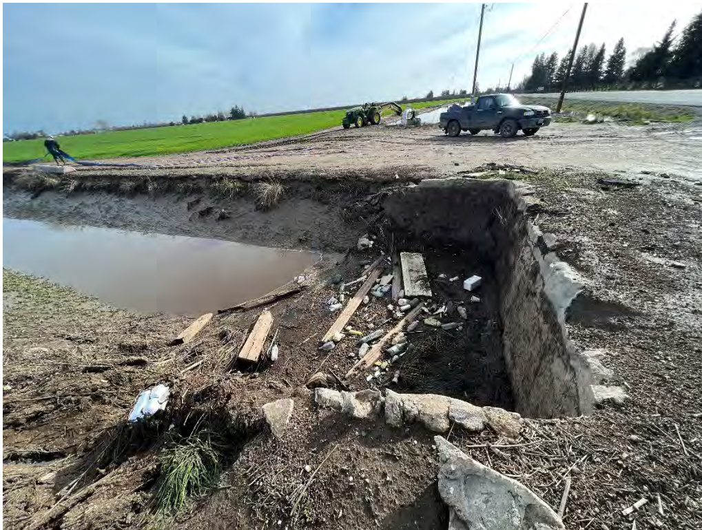
Photograph 40: From the eastern shoulder of Escalon-Bellota Road, looking south at an existing agricultural channel which runs east to west near 12381 Escalon-Bellota Road.
