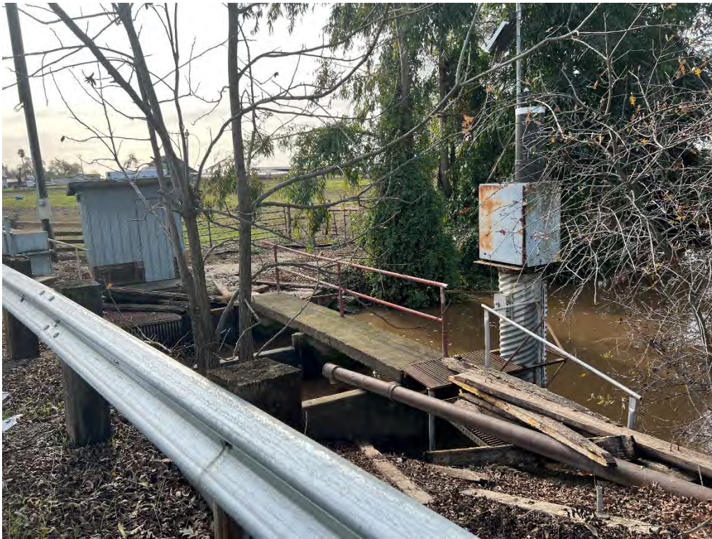
Photograph 19: From the western shoulder of Escalon-Bellota Road, looking southwest at maintenance facilities associated with Lone Tree Creek.
