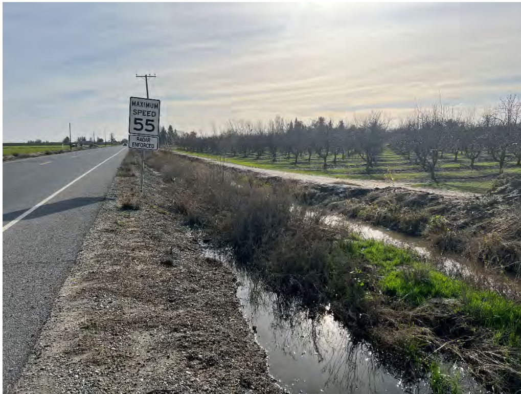
Photograph 44: From the western shoulder of Escalon-Bellota Road, looking south along an existing roadside ditch and agricultural channel located at 12367 County Highway Junction-6 within the proposed project.
