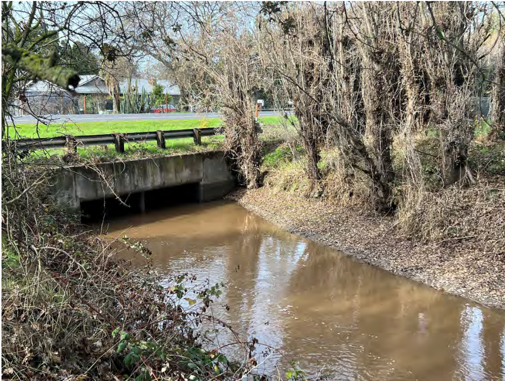
Photograph 18: From the southern bank of Lone Tree Creek, looking northwest toward Escalon-Bellota Road.
