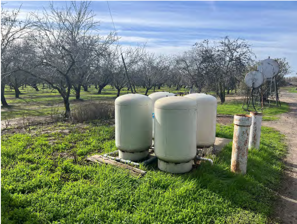
Photograph 7: From an unpaved access road adjacent to the orchard and proposed tank and pump site, looking southwest at existing irrigation tanks.
