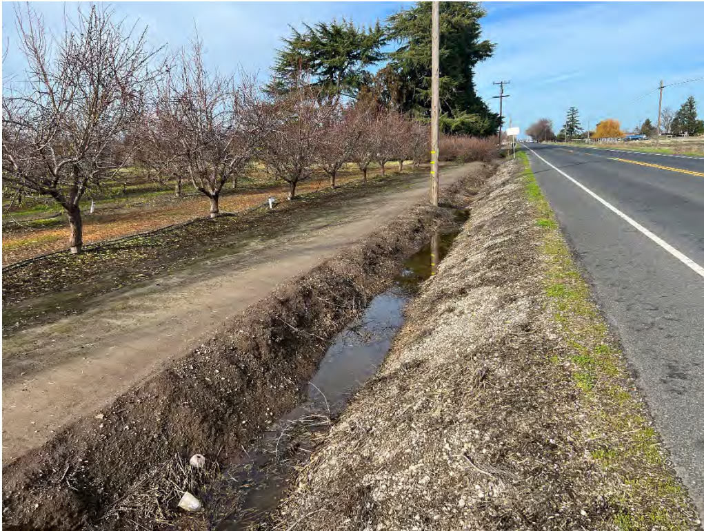
Photograph 31: From the intersection of Escalon-Bellota Road and Edwards Avenue, looking north along Escalon-Bellota Road through a roadside ditch within the project site.
