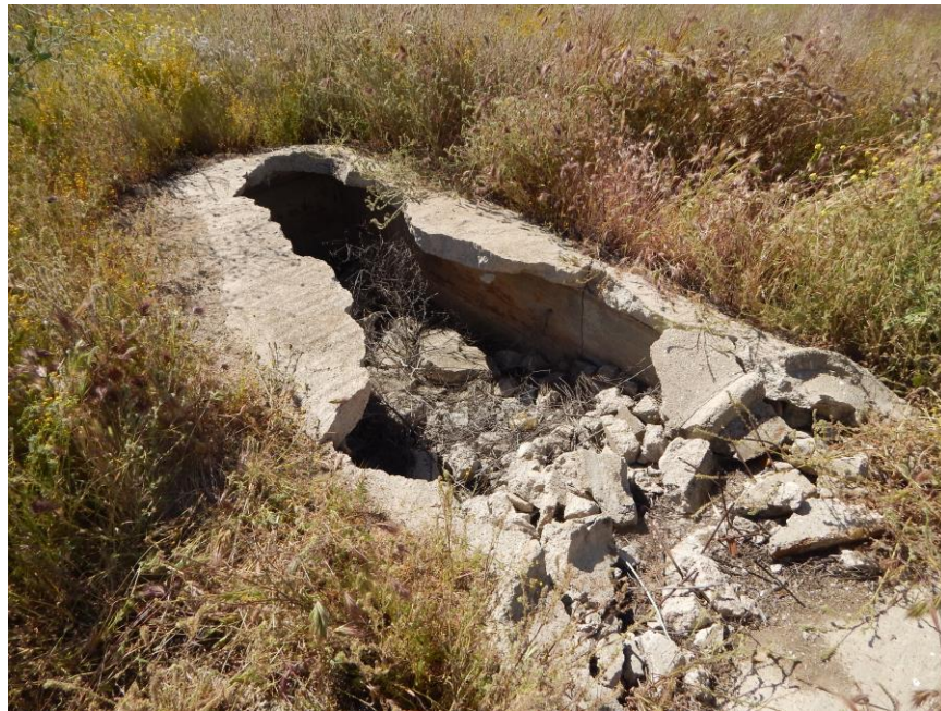
Plate 12. Site P-33-028995, collapsed holding tank of bubbler/guzzler feature, view to the northeast.
