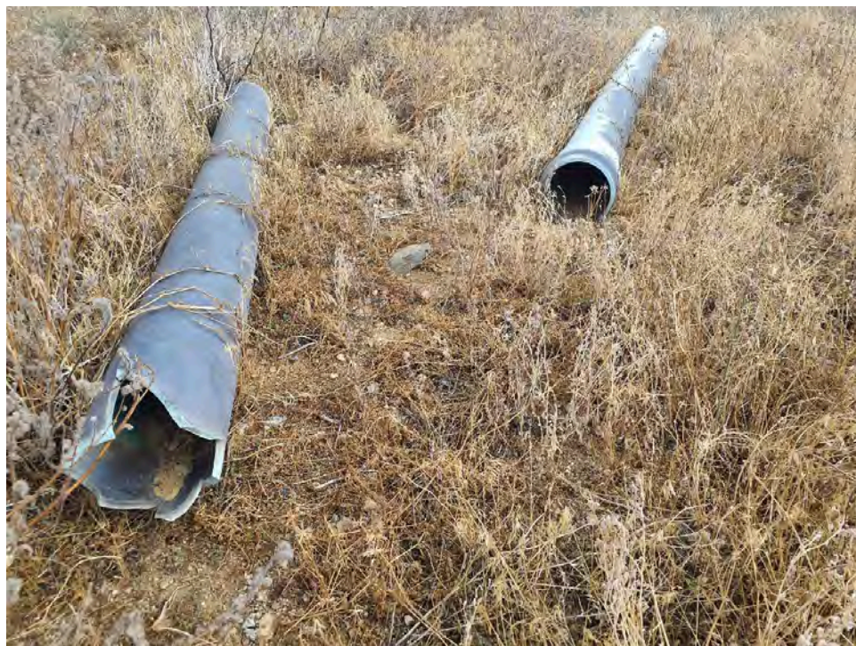
Broken pipe with open ends; good habitat for small mammals, birds, and reptiles.
