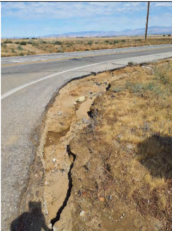
Roadside wash facing north along 70 th Street West.
