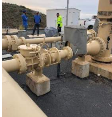
Photo 17: Looking Southeast at the existing pumps and cans.
