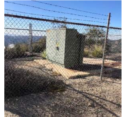
Photo 6: Looking East toward the existing SCE transformer.
