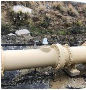
Photo 14: Looking North at the existing surge tank.
