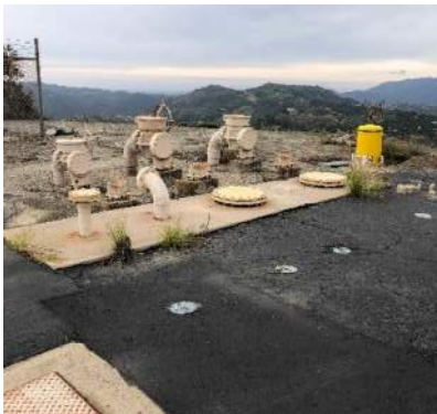
Photo 19: Looking Southeast at the existing pumps adjacent to SCE transformer.
