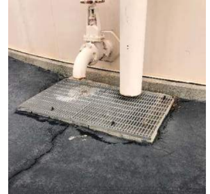
Photo 18: Looking at the external piping at the Carancho Pump Station.
