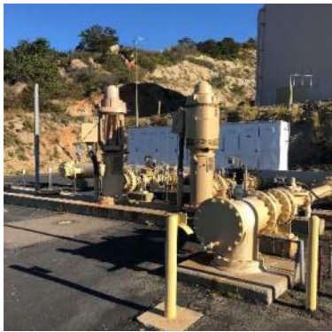
Photo 2: Looking Northwest towards the existing pumps from the lower pad.
