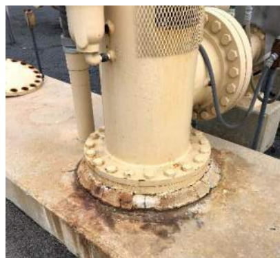
Photo 20: Damage at the existing pump.
