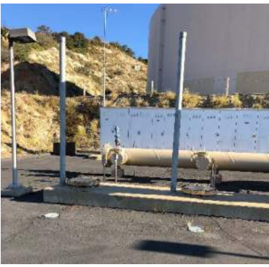
Photo 1: Looking North toward the Electrical Gears from the lower pad.
