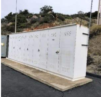
Photo 16: Looking Northwest toward the electrical gears at the lower pad.
