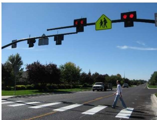
Figure 4: Example PHB Installation
