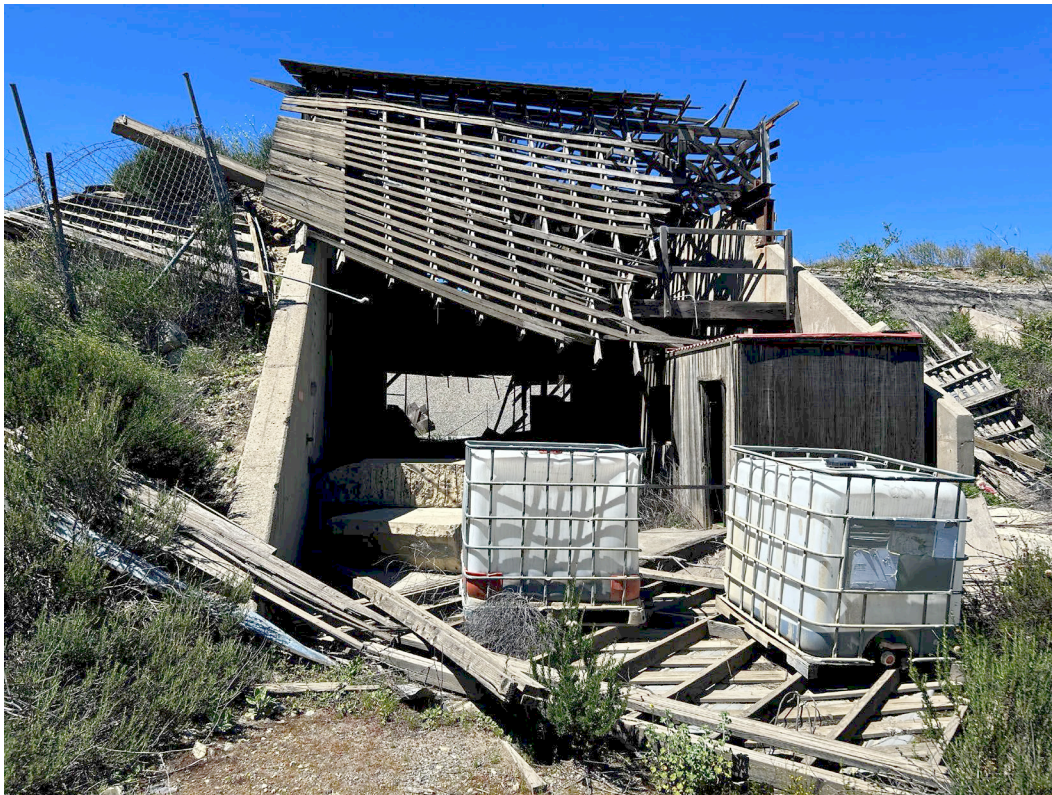
Figure 5: Collapsing Bunker Entrance within Project Area
