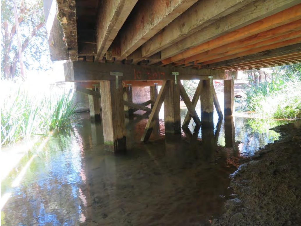
Photograph 7: West-facing view of the underside of the Messick Road Bridge in August 2022, showing inundation of the entire width of Mosher Creek.
