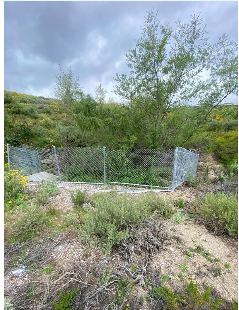
Photograph 8: Northern off-site discharge culvert for Study Area leading into Citrus Heights Residential Development.
