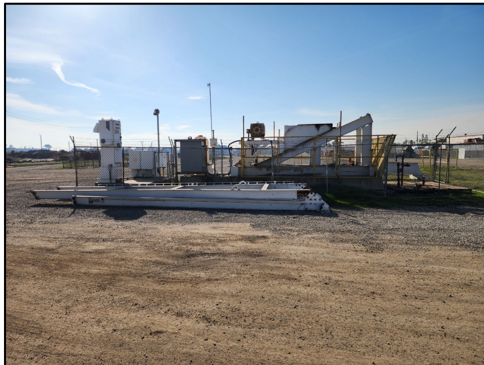
Plate 4: Overview of other equipment found on the subject property, facing east.
