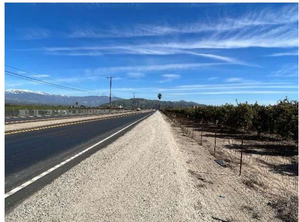
23RW-24 Rose Avenue, 520 ft from South end of RW
