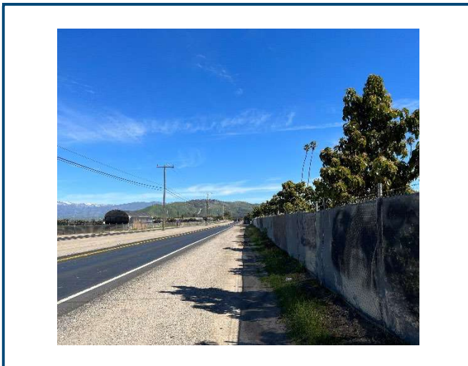
23RW-61 Rose Avenue, 4,280 ft from South end of RW
