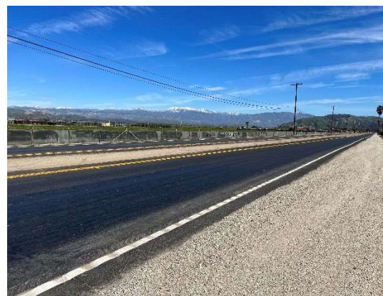
23RW-26 Rose Avenue, Across Oriented N, 520 ft from South end of RW
