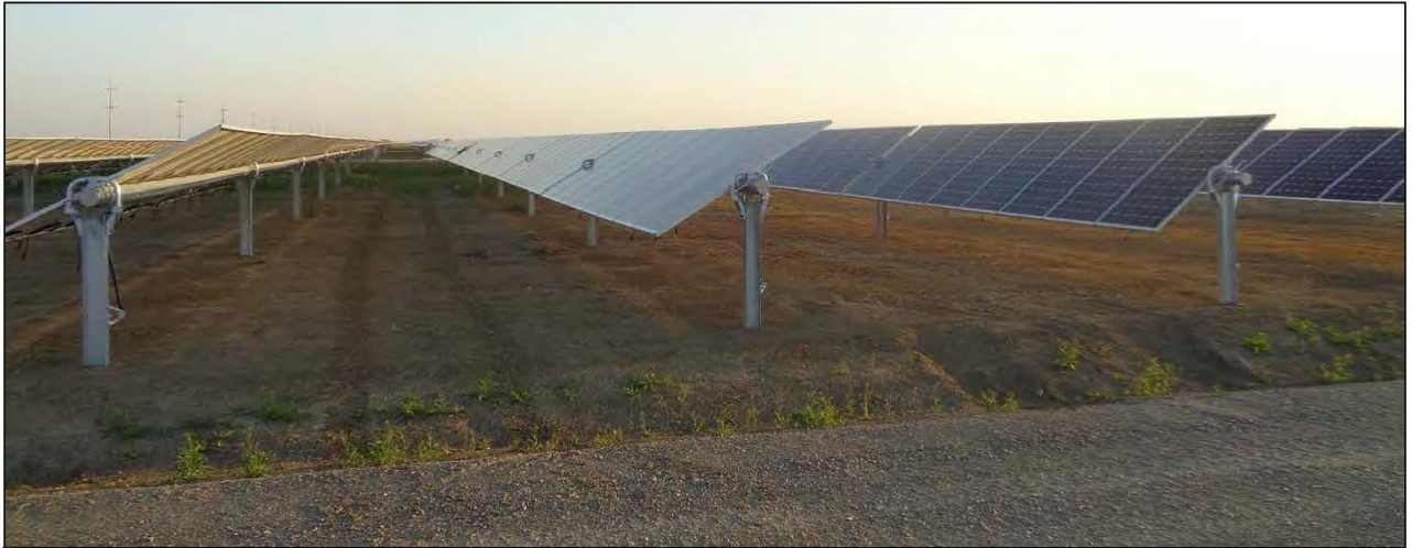
Solar PV Modules on Horizontal Trackers
