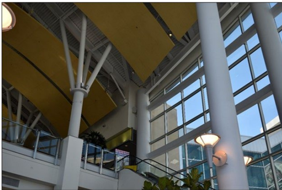
Figure 4 Interior sculptural entrance's roof and connection to the original massing, facing southwest. Source: ICF 2023.
