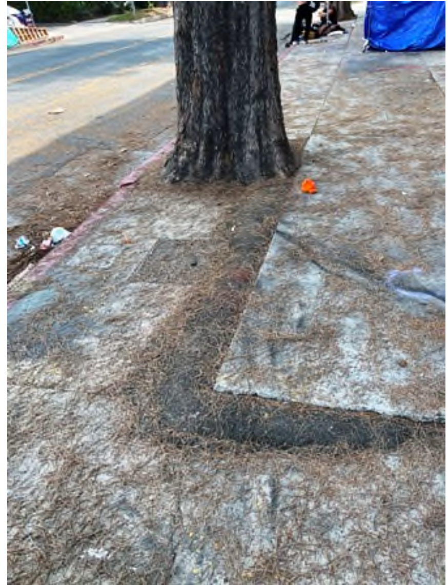
Note its roots lifting the sidewalk
