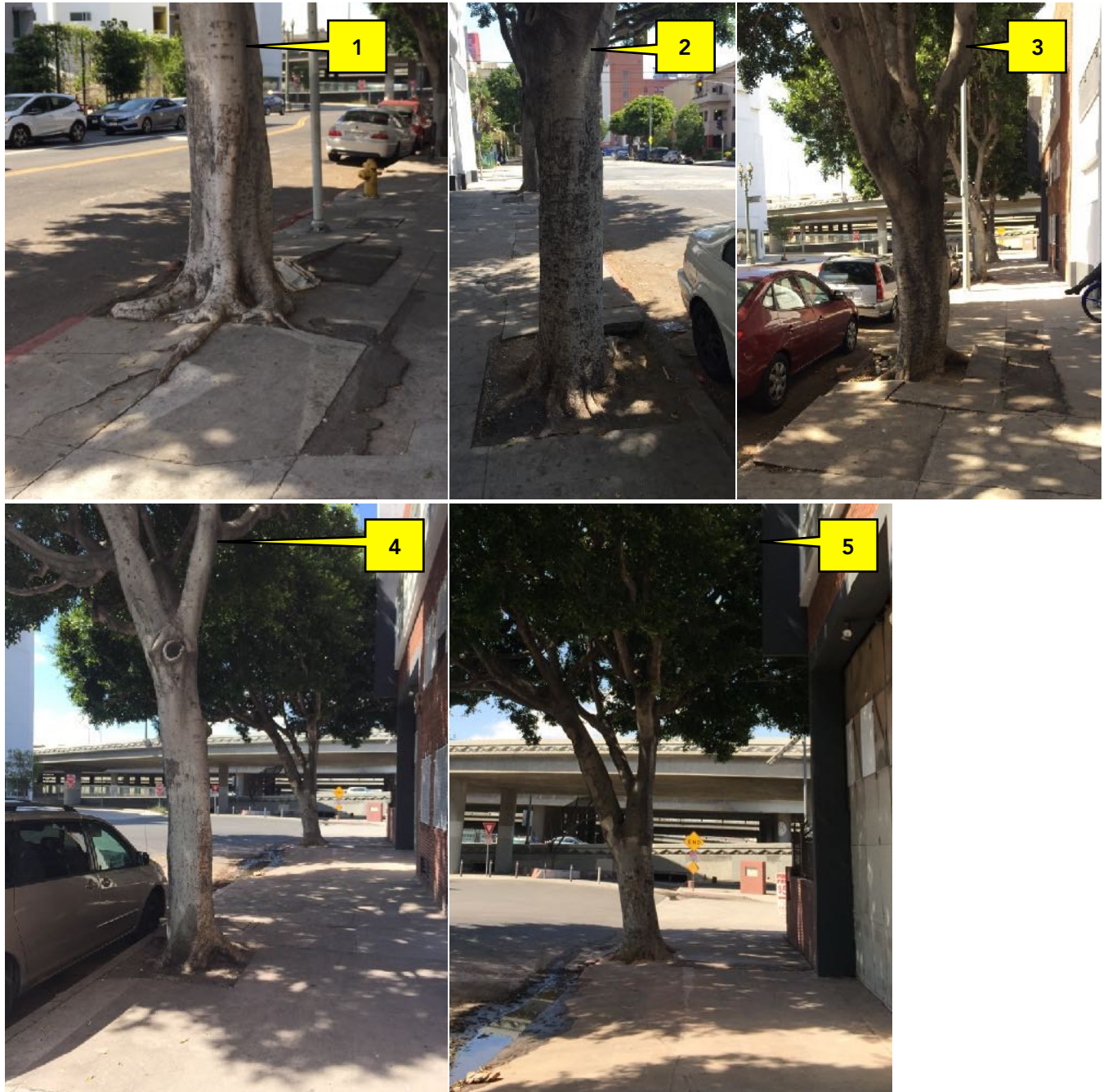
PHOTO 2 - Shows close ups of lifted pavement at the base of Indian laurel fig ( Ficus microcarpa nitida ) street trees #1 - 5.
