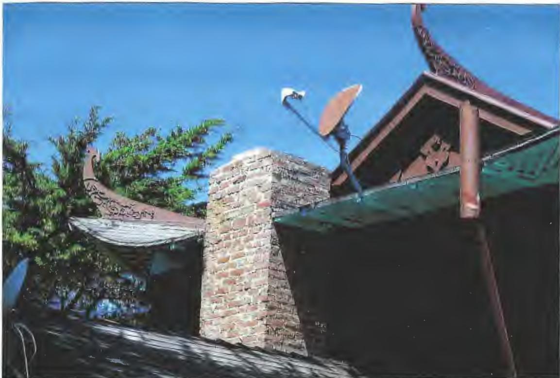
Photo #4. Looking West at the damage done to original roof by, 1950s brick chimney addition, Kent Seavey, December, 2021.
