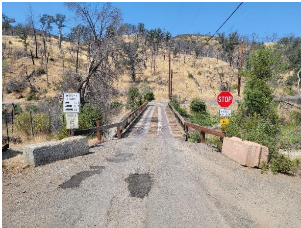
Photo 1: Standing on the east side of the Wolf Creek Bridge looking west.
