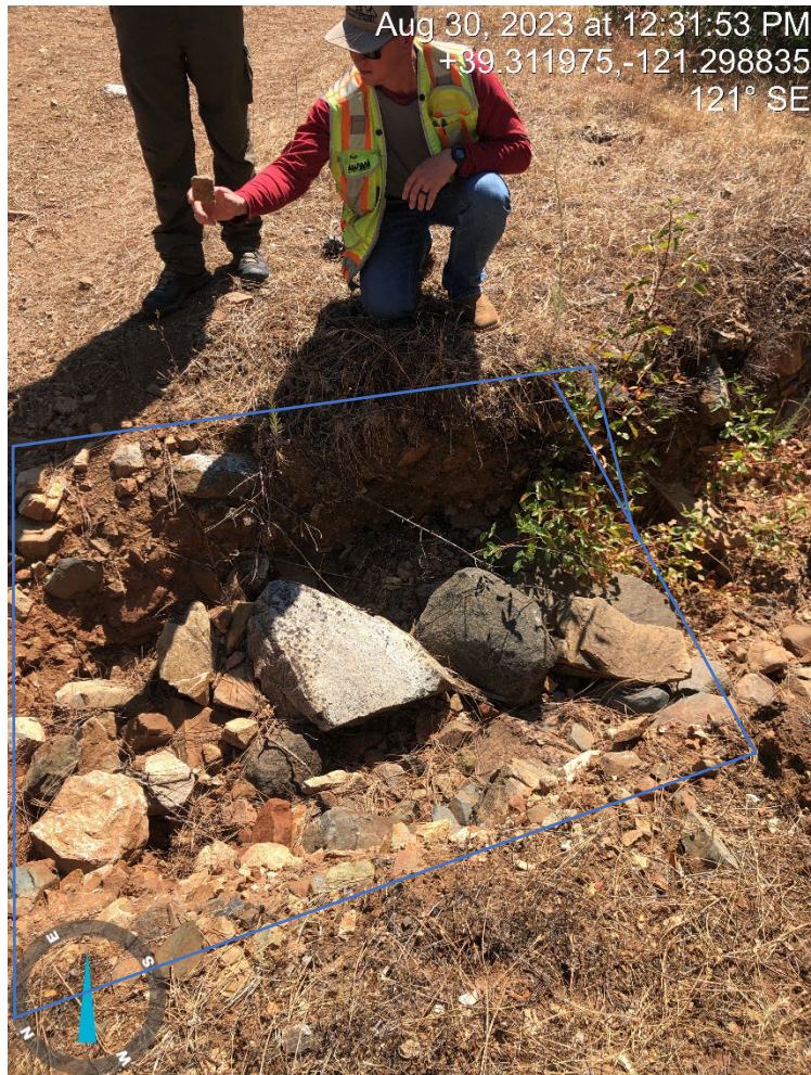
Location 8: Native rocky crossing thru road that has eroded away the fill side of road. Phase 1, install large rip rap armoring to fill in erosion and cap with smaller rock to prevent further erosion (area in blue polygons). No grading or keying in rock will occur.
