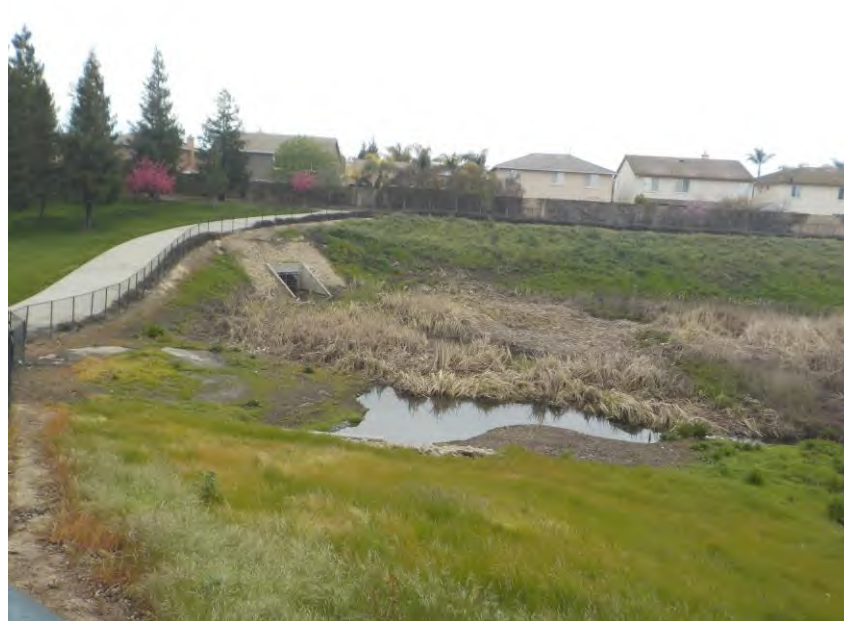
Photograph 6 – View of Concrete Framed Culvert in Northeast Corner of Ustach Park MAR Basin, taken from Northwest Corner, facing East.
