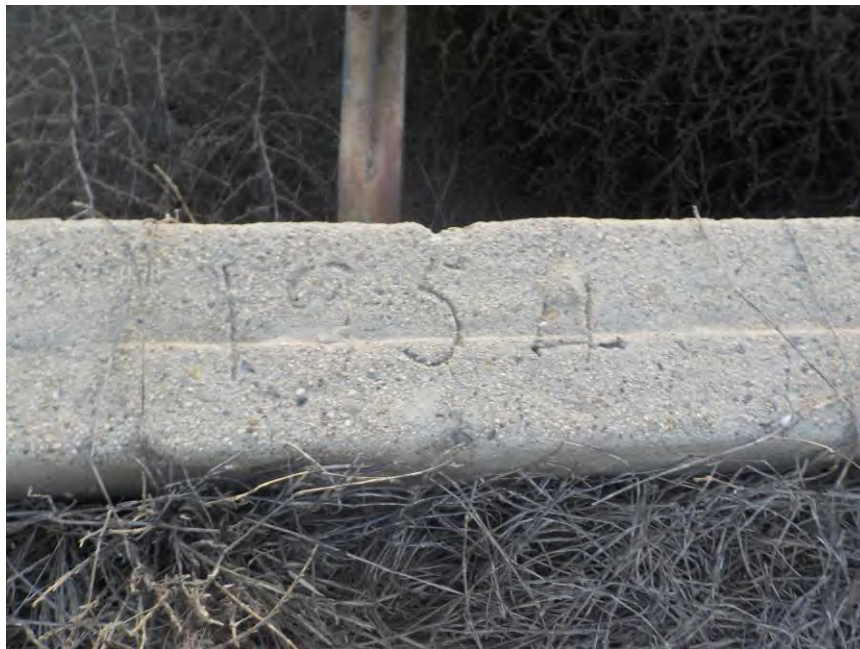
Photograph 18 – Drainage/Irrigation Feature 3, within La Coste Lane Parcel 1 North Mar Basin, Closeup of Top of Northwest Wall, from South, Facing North
