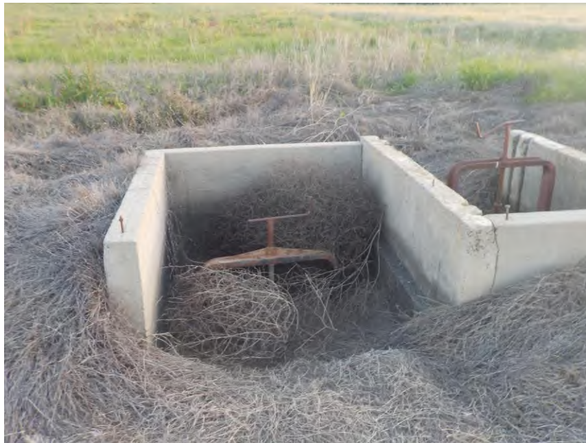
Photograph 16 – Drainage/Irrigation Feature 3, within La Coste Lane Parcel 1 North Mar Basin, from North, Facing South
