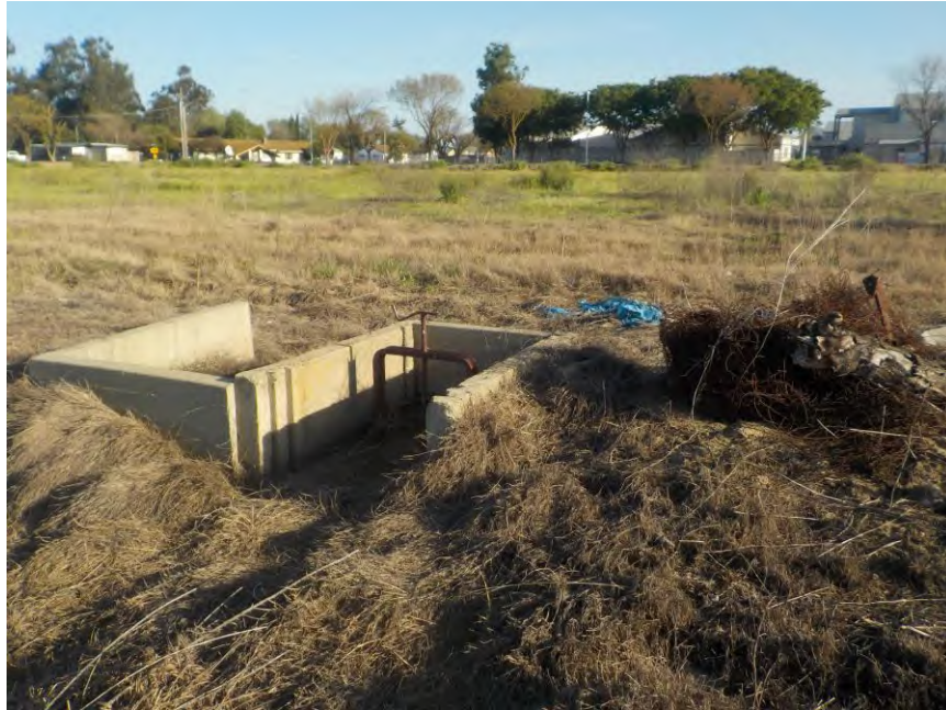
Photograph 15 – Drainage/Irrigation Feature 3, within La Coste Lane Parcel 1 North Mar Basin, from Northwest, Facing Southeast
