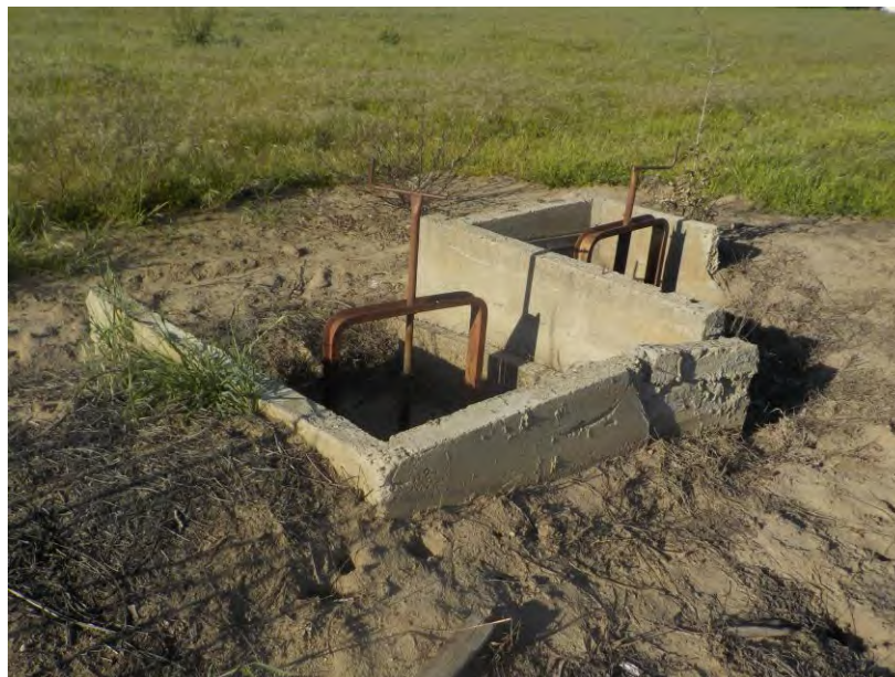
Photograph 10– Drainage/Irrigation Feature 1, within La Coste Lane Parcel 1 North Mar Basin, from Southwest, facing Northeast
