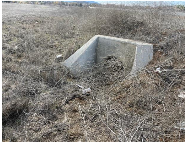
Photograph 2. Storm drainage adjacent to SR 79
