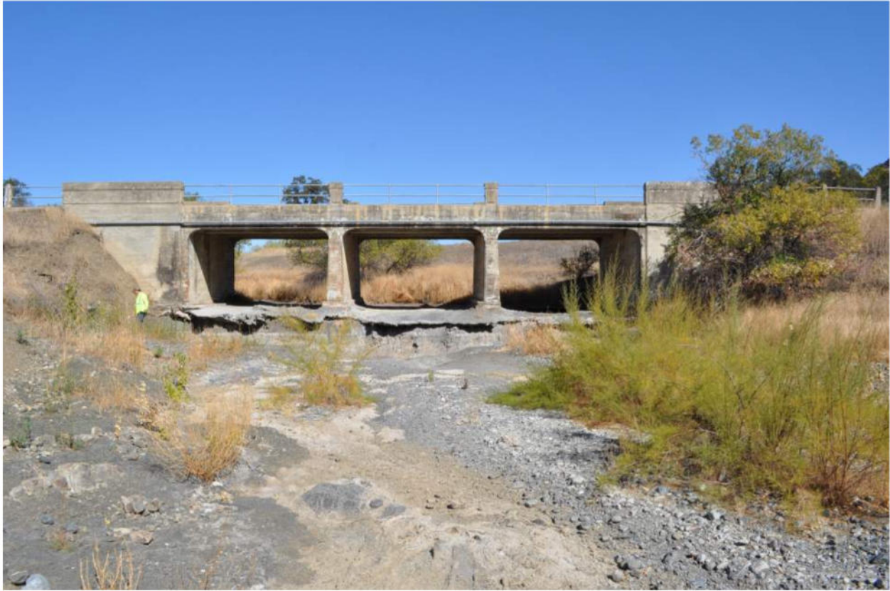
Figure 14. Looking toward the bridge, the concrete lining of the channel is undermined.
