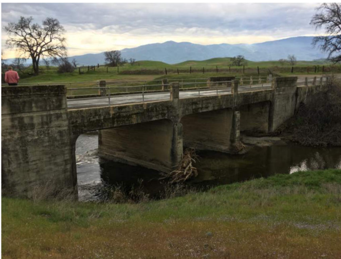
Figure 12. Drift and debris on both piers of the existing bridge
