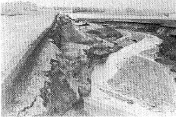
Figure 19 — Extensive channel erosion took place on Hicks Canyon Wash, at Jeffrey Road, during the flood of February 1969. A portion of the improved gunite channel still remains (upper center of photo) several feet above the new channel invert. (Photo courtesy of the Irvine Company.)
