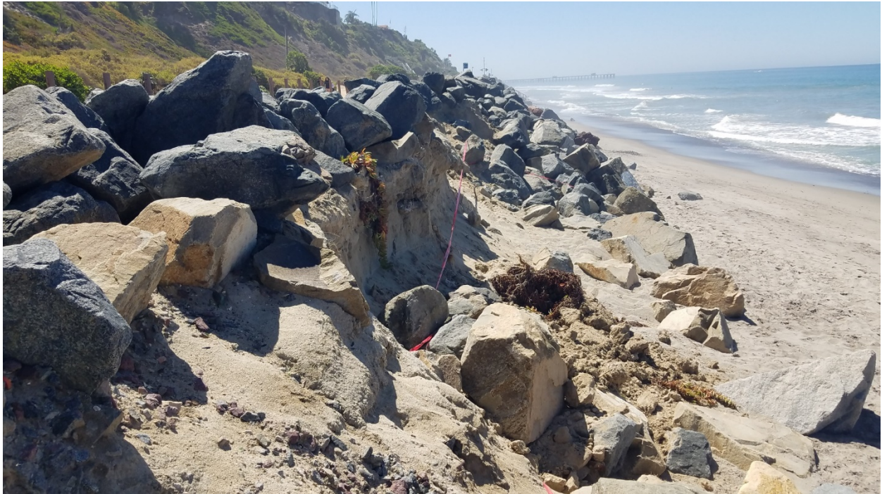
Damage to Revetment:
