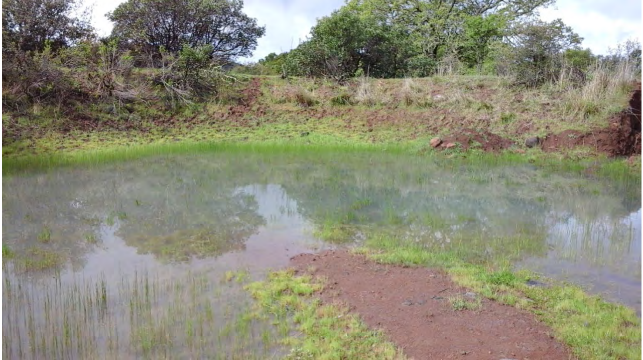
Photo 3. Looking west at the breached stock pond. Photo date April 2017.
