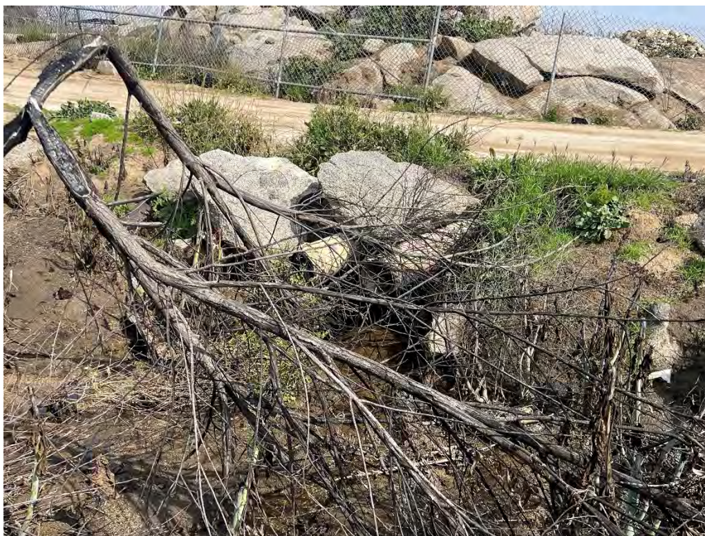
Photograph 4: Drainage A terminates at two culverts that convey flows beneath the unnamed access road that bounds the eastern boundary of the southern portion of the project site.
