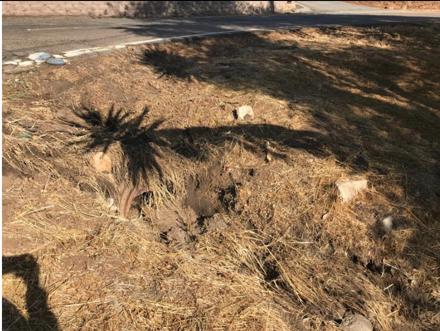
Photograph 1: (33.194999 N, -117.240876 W) Northwest-facing view of the western reach of the two-foot-wide Channel 1 in the western portion of the Project site. This photo also shows where the highly eroded channel forms at the outlet of the two-foot-diameter corrugated metal culvert on the western edge of the Project site. This photo shows where Sampling Point NW-1-1 was taken to determine the presence of OHWM indicators. This photo also shows the sediment clogging the corrugated metal culvert and the erosion of the channel at the outlet of the culvert.
