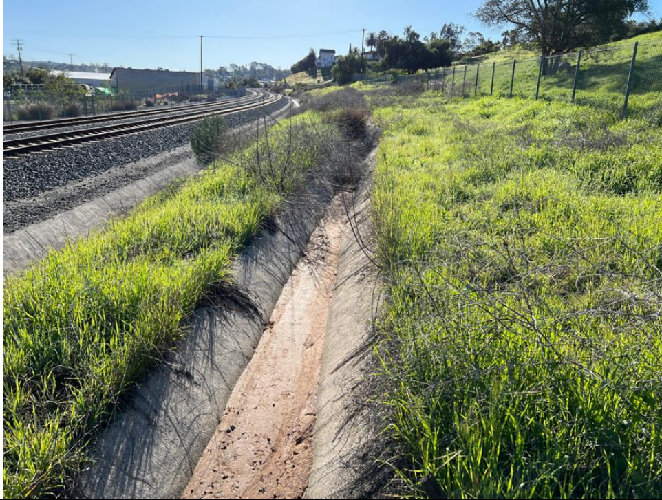
Photograph 11: (33.196216 N, -117.240421 W) Southeast-facing view of Channel 3. This photo shows the upland grasses and weeds growing outside of the channel banks. The eastern side of the Project site and the chain-link fence separating it from the eastern portion of the survey area is visible in the upper right-hand-corner of the photograph.
