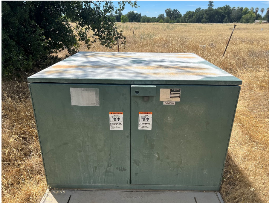
Photograph 16, view facing west: Electric transformer box located at the east edge of the Subject Property.
