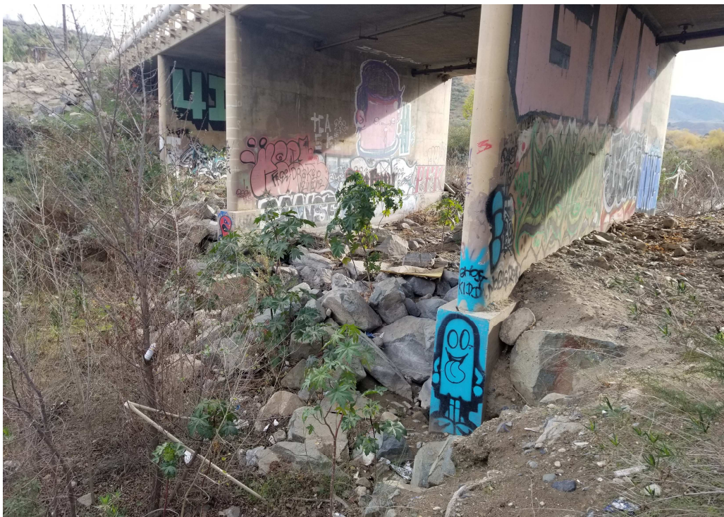
Photograph 6: Downstream-facing view of Dawson Canyon Bridge piers from the northeast end of the bridge. The terrace on the right (northeast) side of the photo is above Corps and CDFW jurisdiction. The northeastern-most pier is not pictured but is to the right (northeast) of the piers in the photo and is above jurisdictional limits of both Corps and CDFW.
