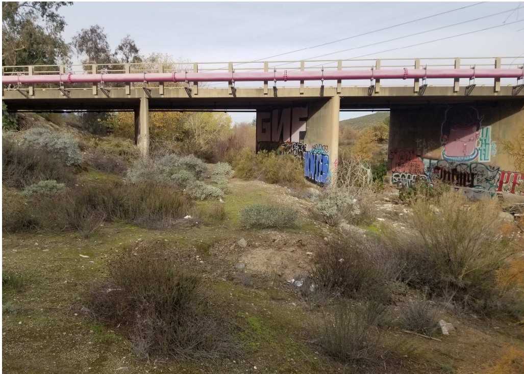
Photograph 5: Downstream-facing view of Dawson Canyon Bridge piers on the southwest end of the bridge. The southwestern-most pier is on an upland terrace above CDFW and Corps jurisdiction.
