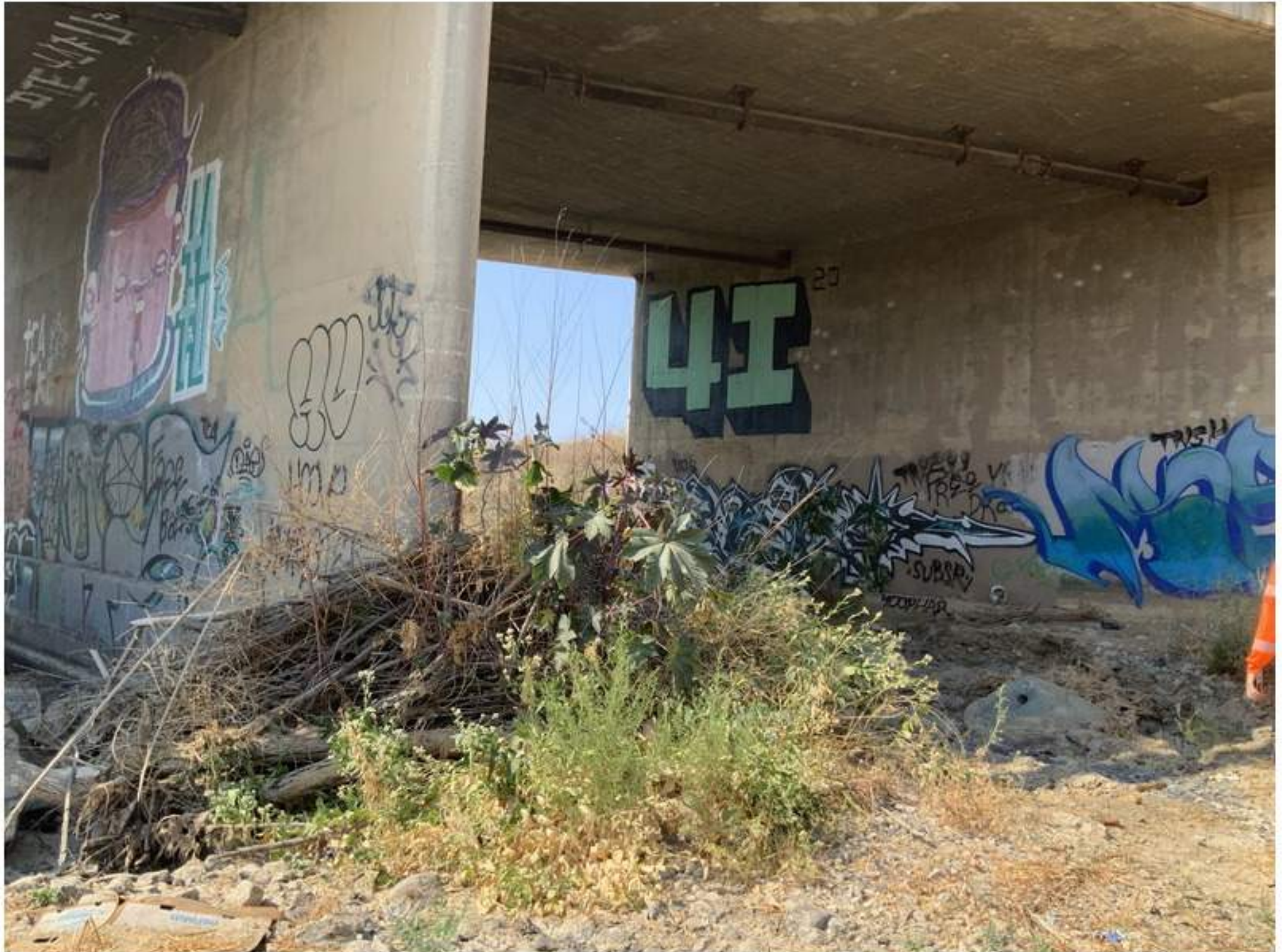
Photo No. 108 Debris At The Pier
