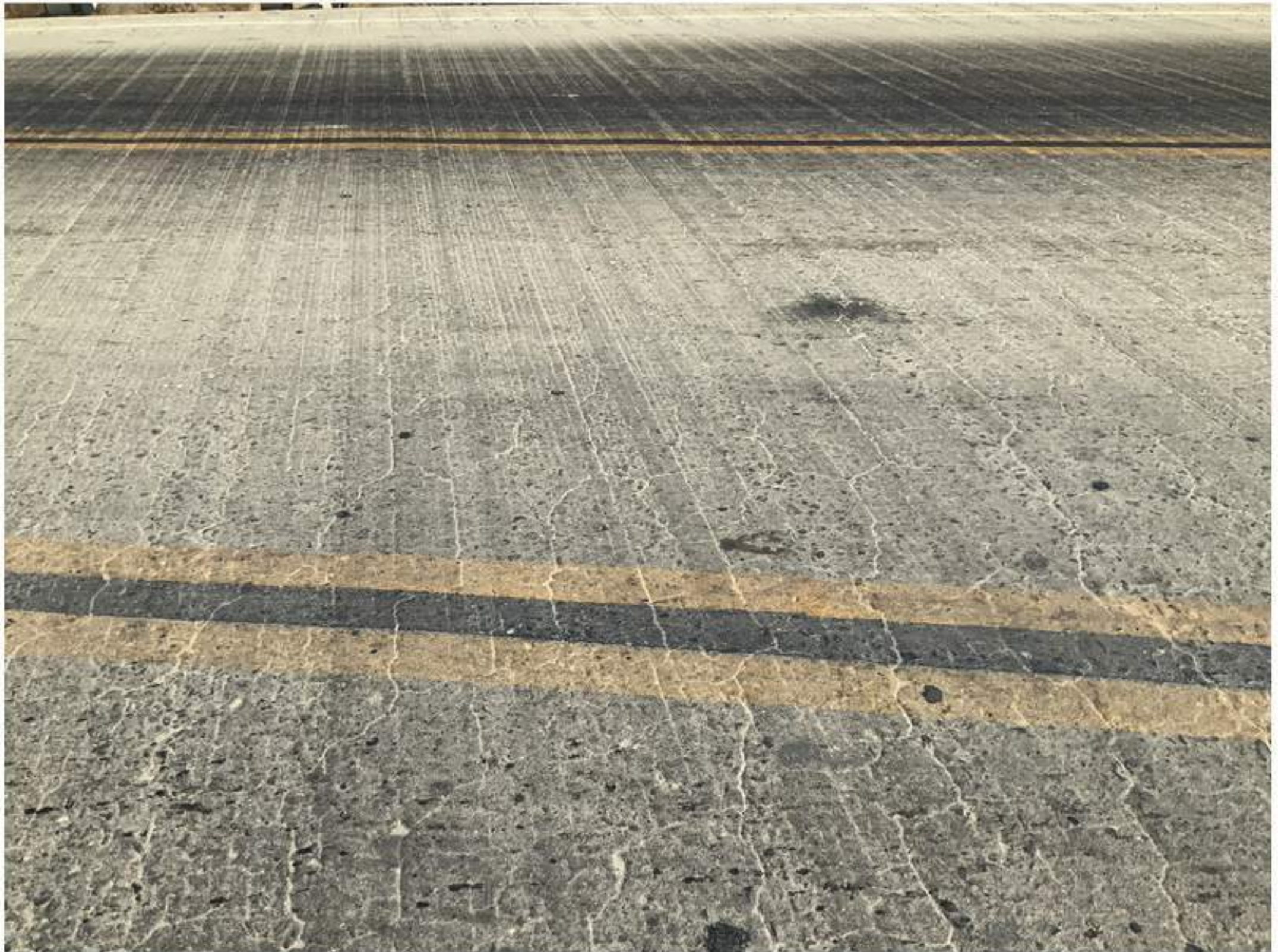
Photo No. 104 Typical Deck Cracks
