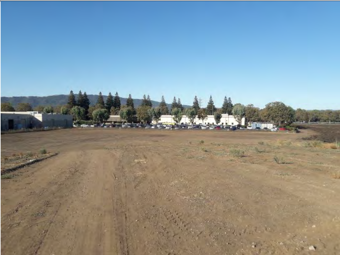
Photograph: 7 View of the graded area west of the southwest portion of the Site. The Kaiser Permanente medical office building is visible in the background.
