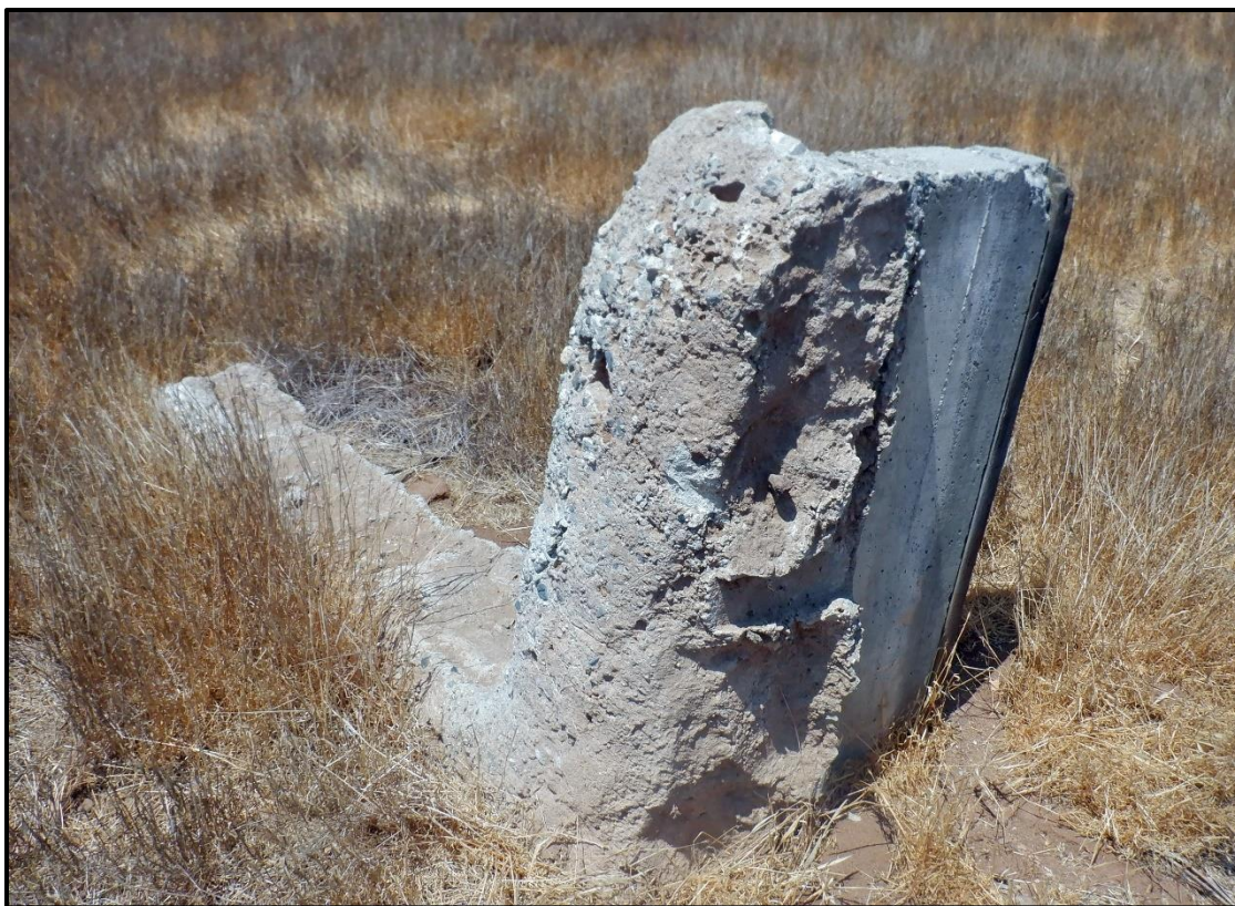
Figure 23. Displaced Segment of Concrete Foundation.
