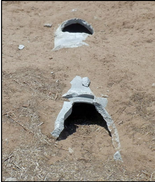
Figure 18. Example of Irrigation Pipe.
