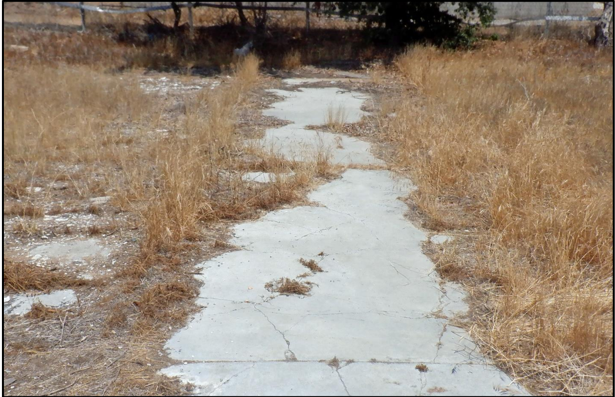
Figure 26. Concrete Walkway along a Broken and Semi-Demolished Concrete Pad (NE).
