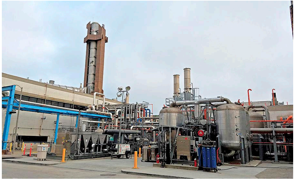
Water/Environment - Award of Merit South: Digester Gas Utilization Project. The tight deadline for this digester gas cogeneration facility required the use of a design-build-operate delivery method not traditionally used by the city.
