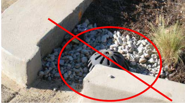
Figure 6: Incorrect Placement of an Overflow Inlet.
