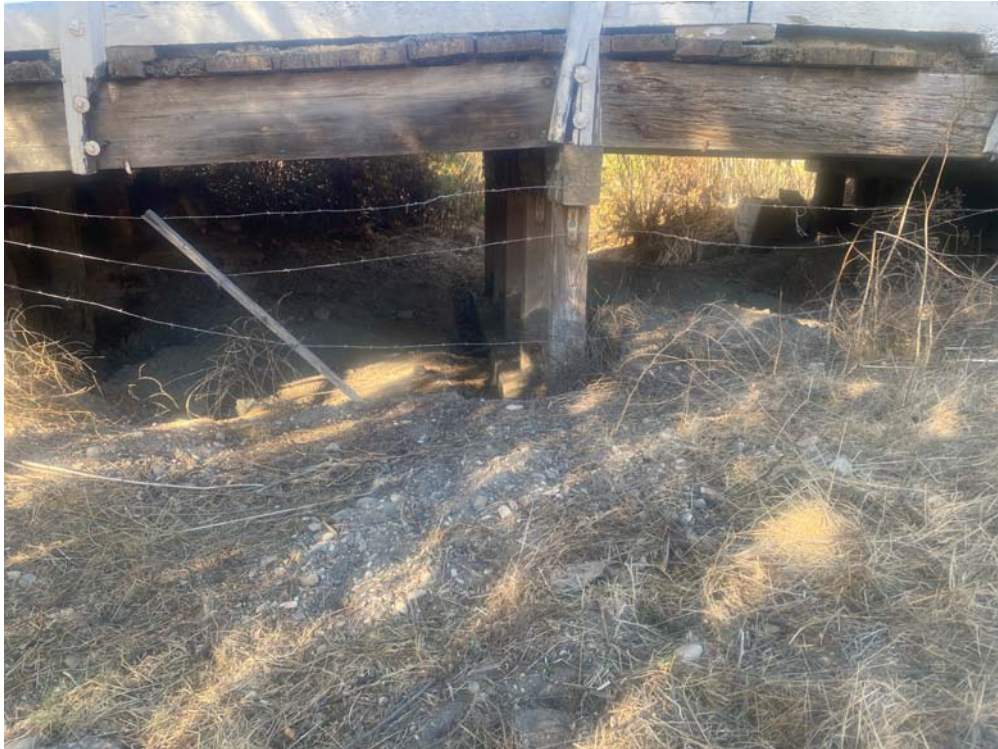
Photo 7. View under the bridge showing structural issues and sedimentation around the piers.
