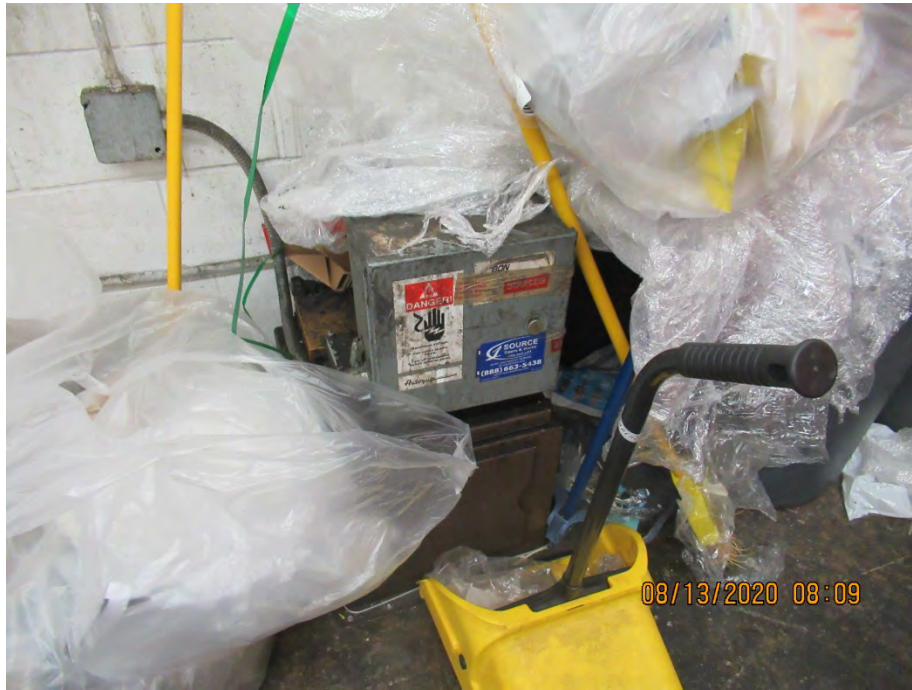
15. Loading dock plate hydraulic equipment.
