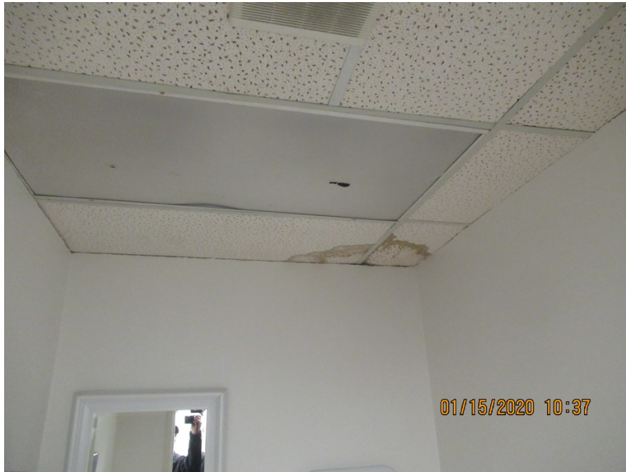
19. Water-stained ceiling tiles.
