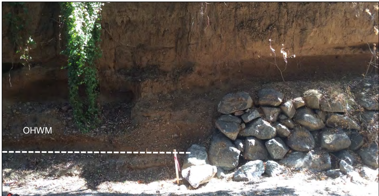
Photograph 12. An OHWM scour line (bottom left) along the steeply eroded east bank corresponds with the elevation of a break in bank slope on the opposite bank at OHMW Transect 4. Directly upstream is a reach of rock rip-rap bank stabilization.
