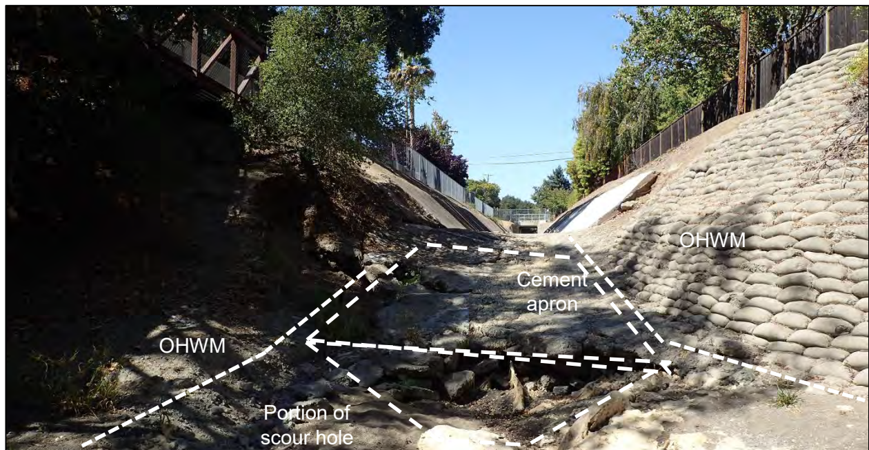
Photograph 8. The confluence of Regnart and Calabazas Creeks, viewed from Calabazas Creek facing west. At Regnart Creek, above the cement lined banks, bare earth banks rise to the top of bank. Regnart Creek is approximately eight feet higher than Calabazas Creek and a cement apron connects Regnart Creek to Calabazas Creek, below which a scour hole (bottom) has developed in the Calabazas Creek bed.
