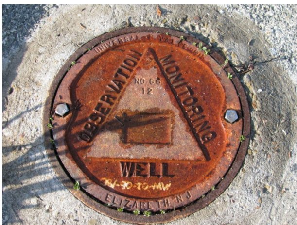
PHOTO 3.3: View of cap plate for on-site monitoring well
