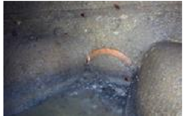
Line From East Plugged
