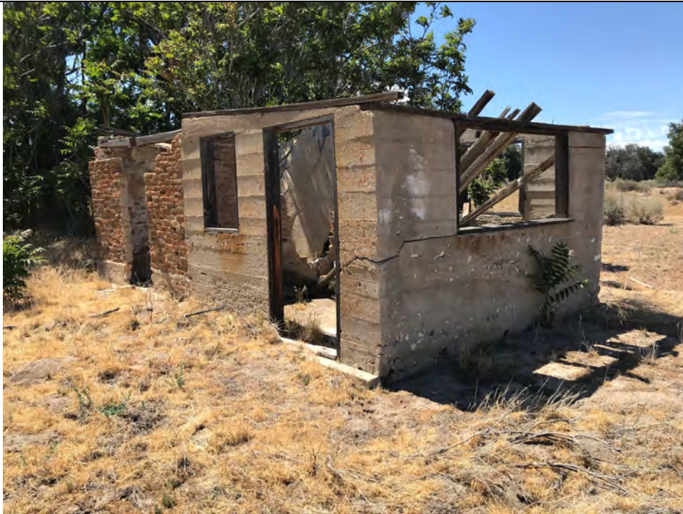
Photo 45. Old residence with collapsed roof. No utilities found.
