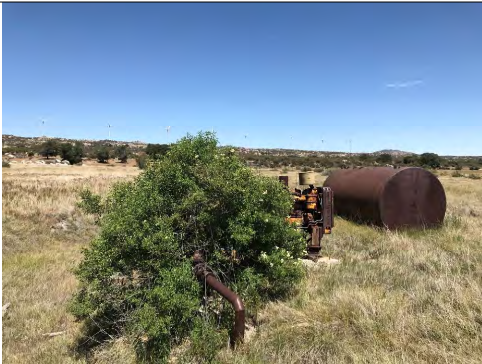
Photo 23. Larger motor and AST with second well south of the smaller well. Well was covered by a bush. Label on AST was rusted over but appeared to be roughly 3-4,000 gallon capacity.
