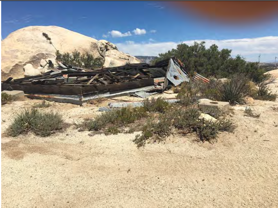
Photo 28. Collapsed house/structure near the observation well.
