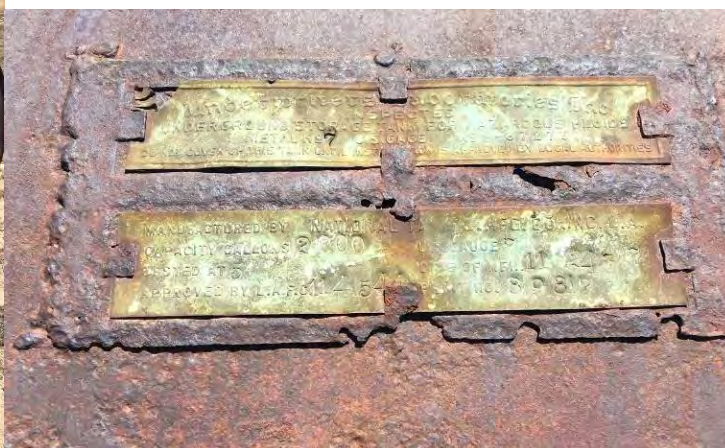
Photo 21. AST had open ports at the top with petroleum odors and visible liquid at least half way down. The label indicated a 2000 gallon capacity.
