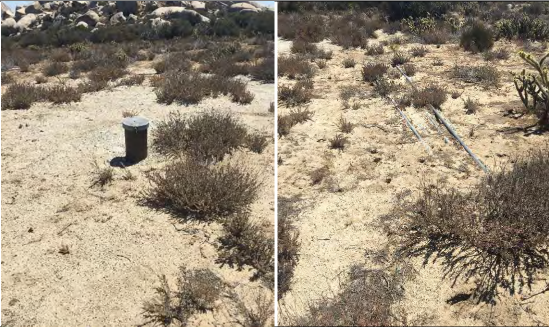
Photo 26 (left). Observation well with locked cap in northeastern end of property. Photo 27 (right). Disconnected metal piping near the observation well.
