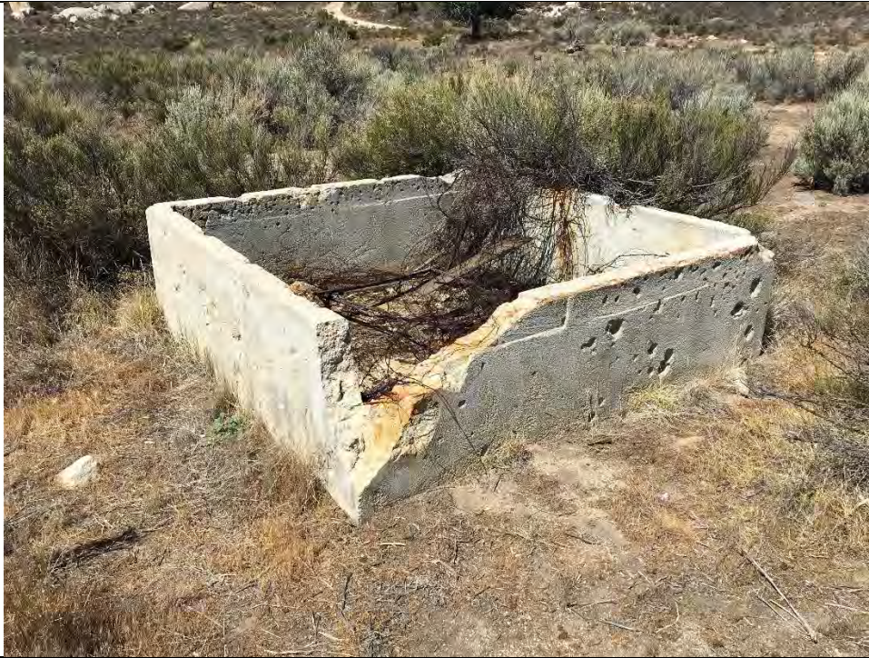
Photo 31. Possible cistern 5' x 5' and about 2' tall. Broken glass, wood planks and metal wiring inside.
