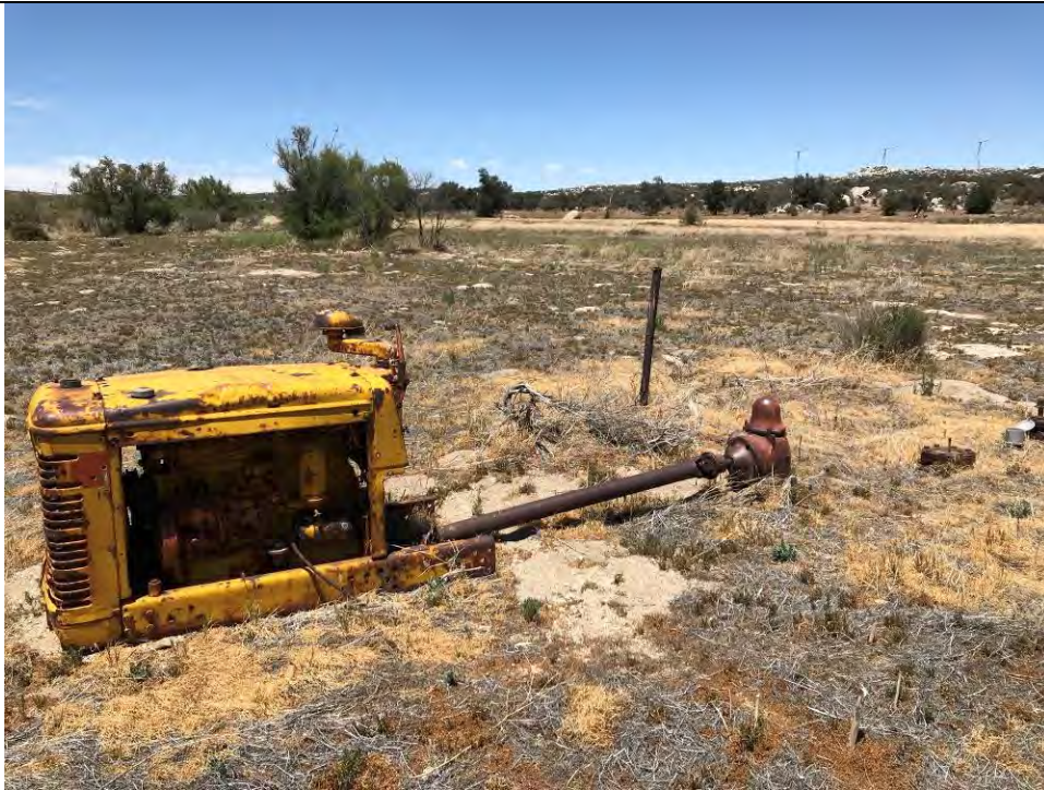
Photo 22. Well and pump assembly. Vegetation near pump appeared stressed based on yellowing.
