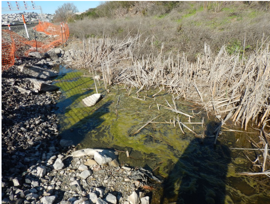
Figure 26 Ponding water, algae and cattail in SPN-2003-280500-W-18
