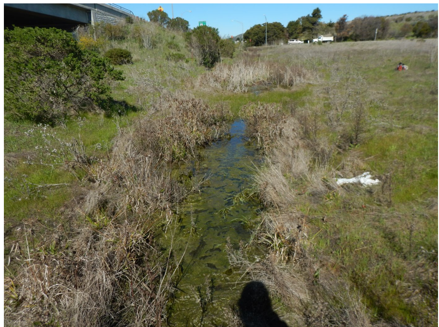
Figure 33 Ponded water in SPN-2003-280500-W-28
