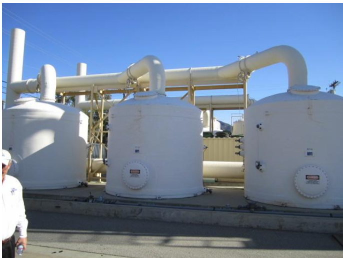
Photo 2. One train of VPGAC units
