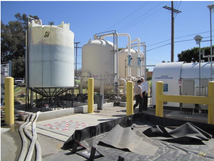
Photo 31. Well-head WBA process at GS-3
