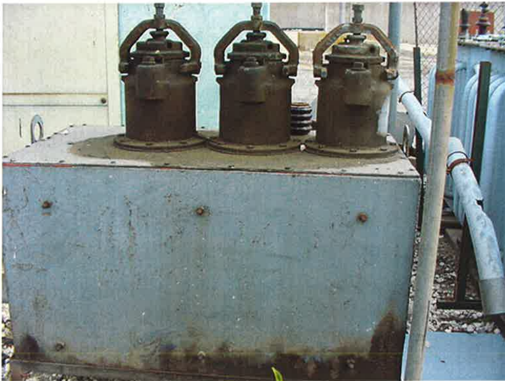
Capacitor bank (typical).
