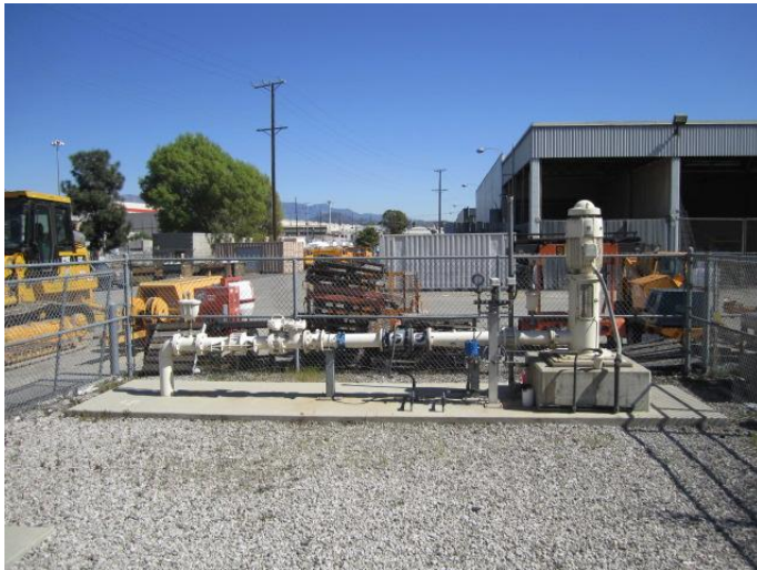
Photo 28. Extraction well GS-1
