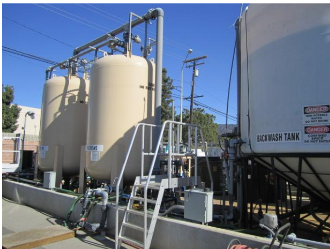
Photo 19. More RCF system components
