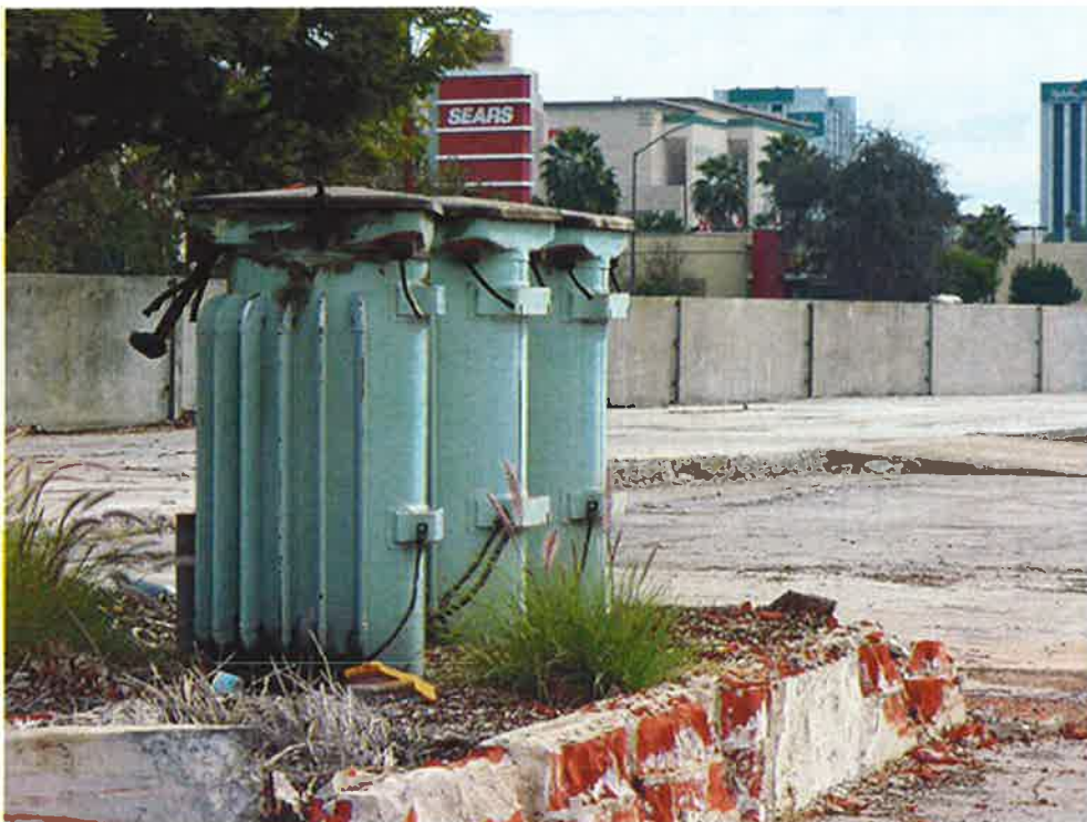
Transformers in former northwest substation.
