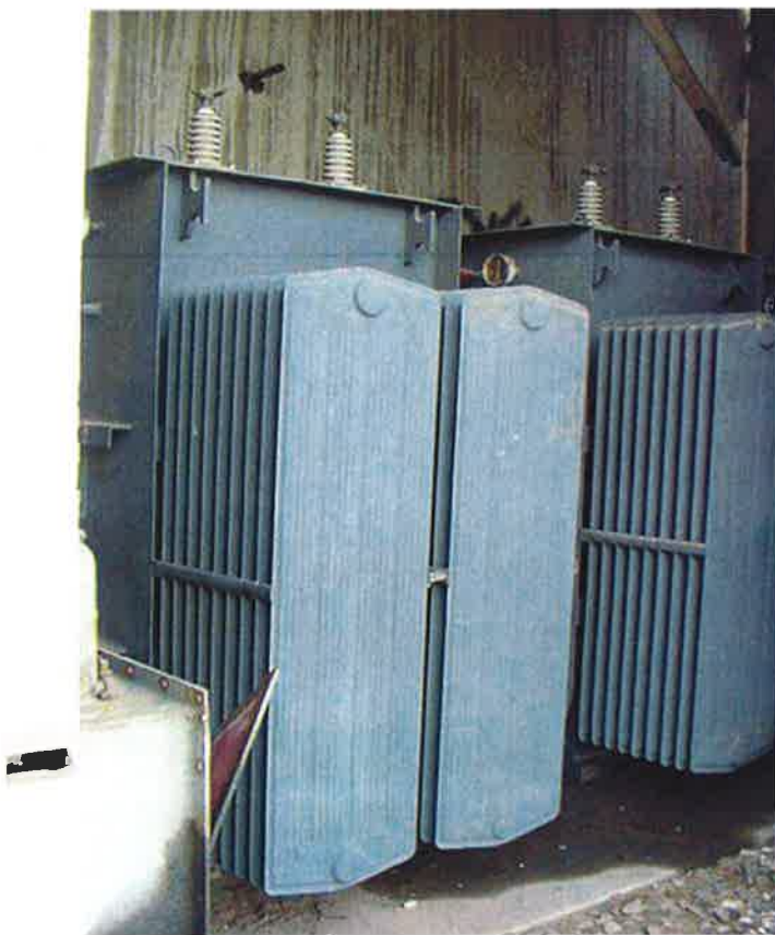
Transformers in eastern substation. Note staining on concrete and gravel.
