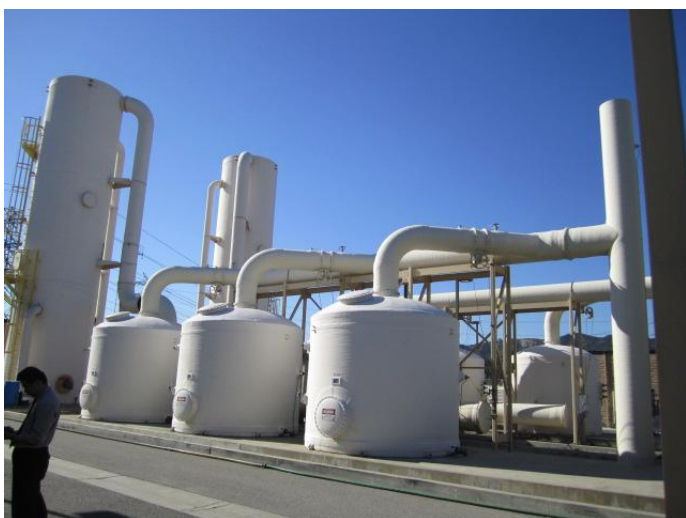
Photo 6. Air strippers and VPGAC units
