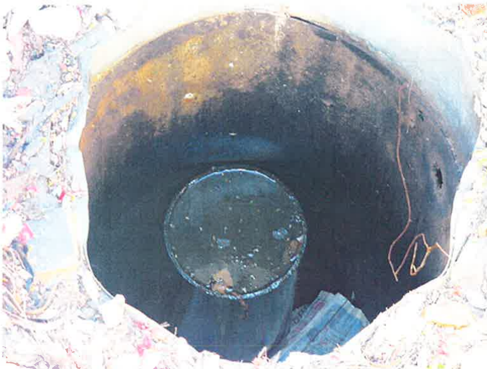
Hydraulic cylinder in base of elevator pit.
