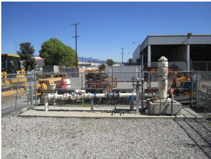
Photo 28. Extraction well GS-1
