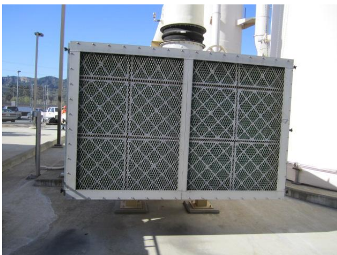
Photo 7. Air intake/filter for air stripper
