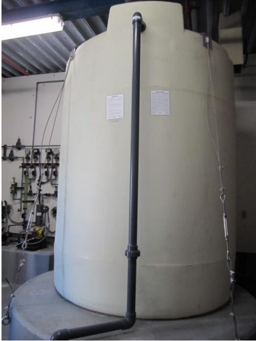
Photo 15. Sodium hypochlorite storage tank
