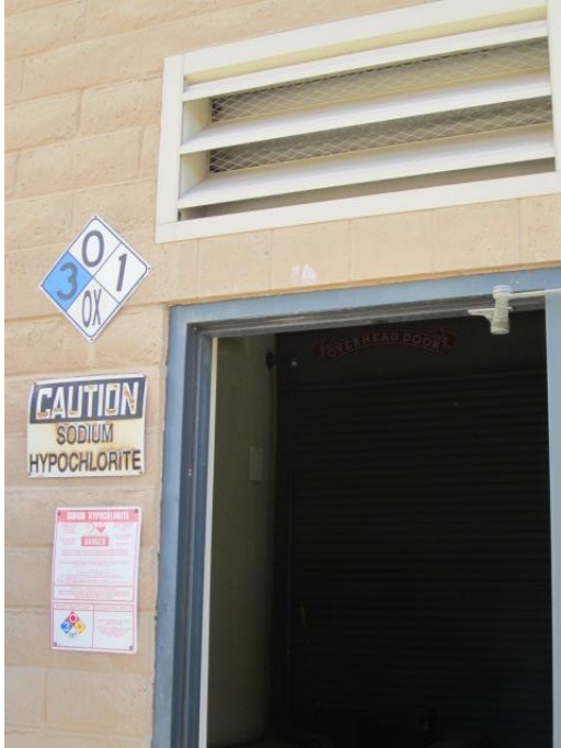
Photo 13. Sodium hypochlorite feed room entrance
