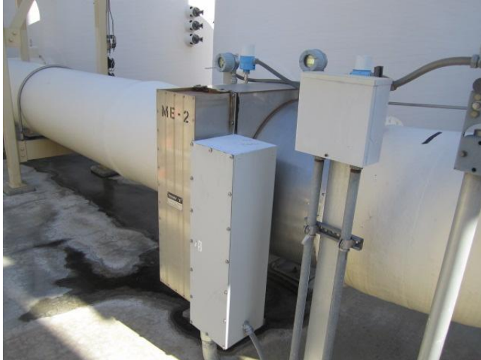
Photo 17. Heater upstream of VPGAC units
