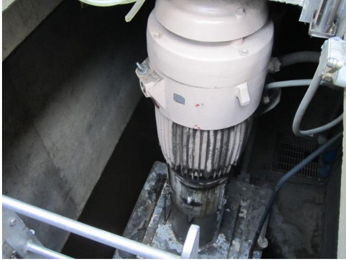
Photo 22. Extraction well GN-4 (from outside the vault)
