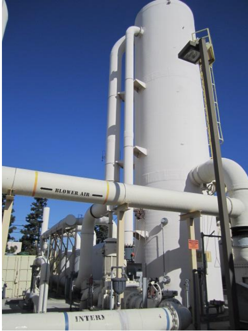
Photo 3. One train (air stripper and three VPGAC units)
