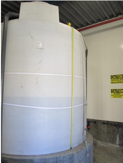
Photo 11. Anti-scalant storage tank
