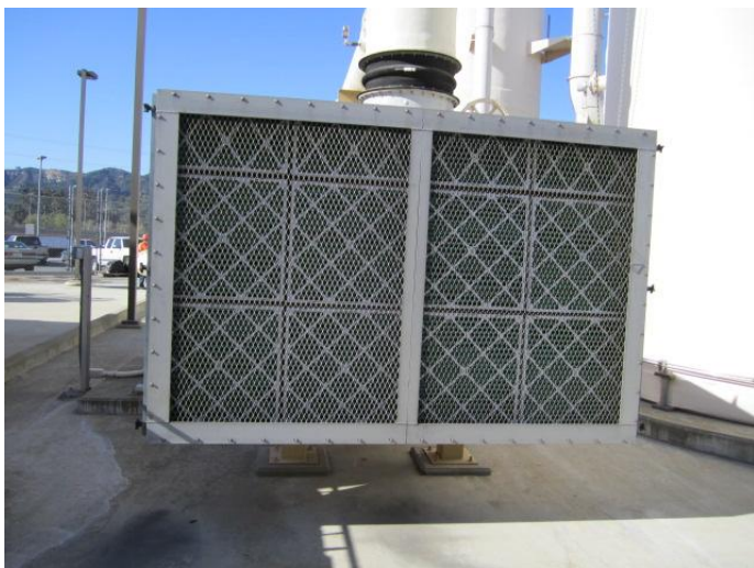
Photo 7. Air intake/filter for air stripper
