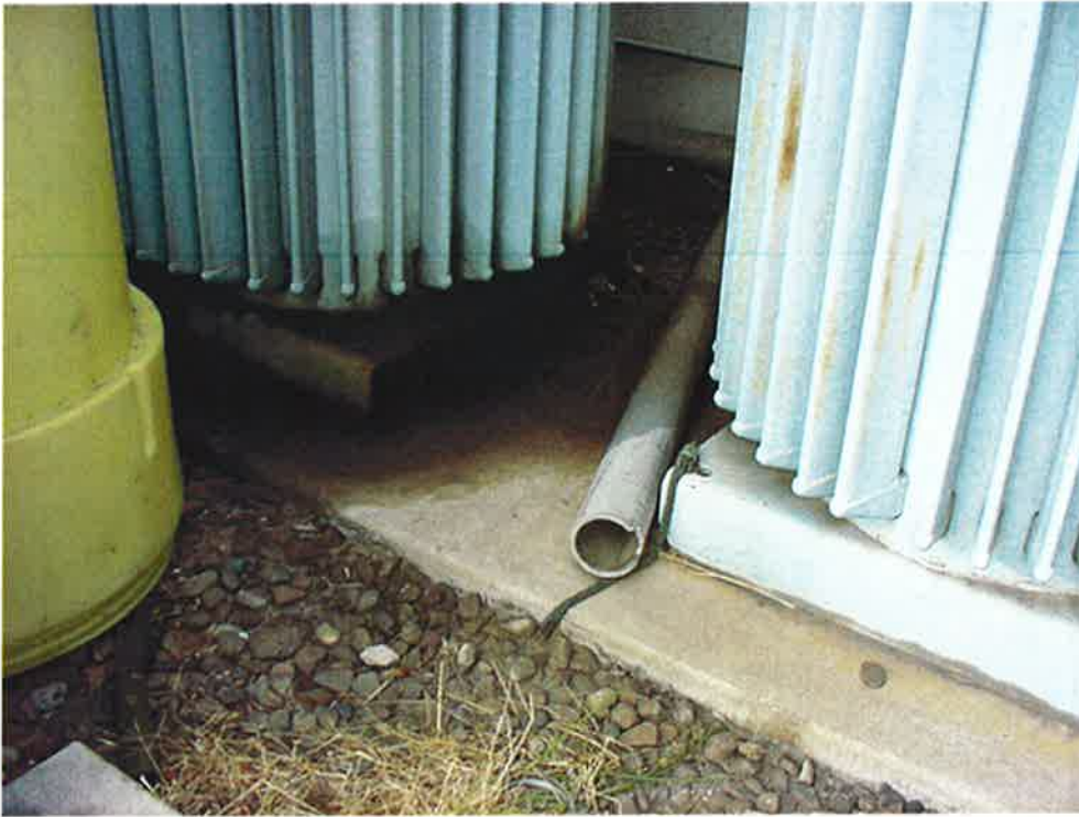
Example staining on concrete and gravel surfaces (typical).
