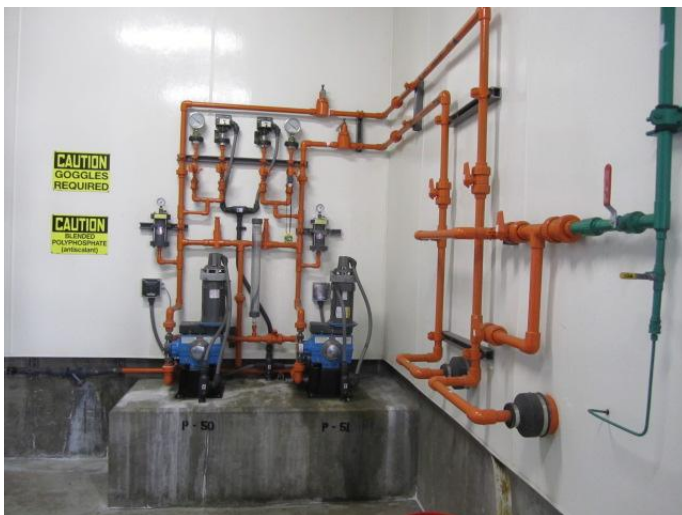
Photo 10. Anti-scalant chemical feed
