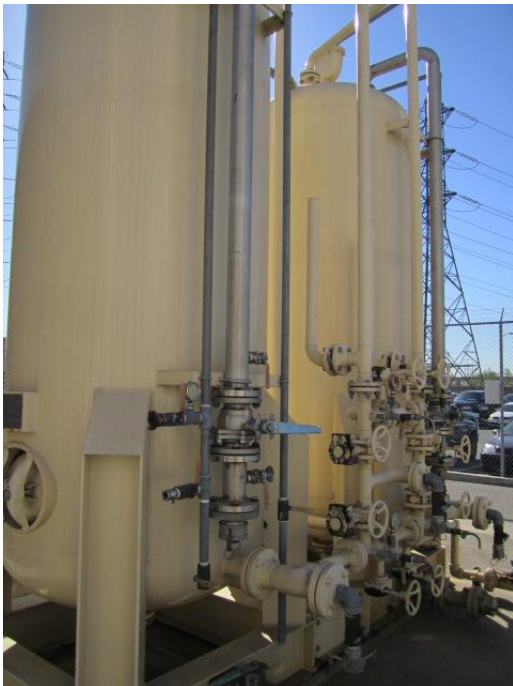
Photo 16. Stormwater treatment system
