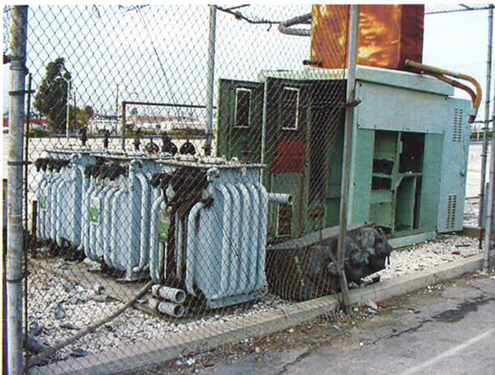
Transformers in central substation.
