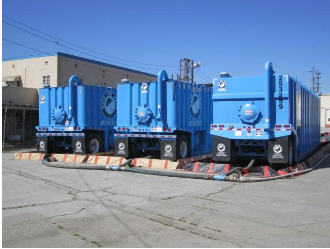
Photo 32. Water storage units for degradation of formaldehyde from initial flushing of ion-exchange resin
