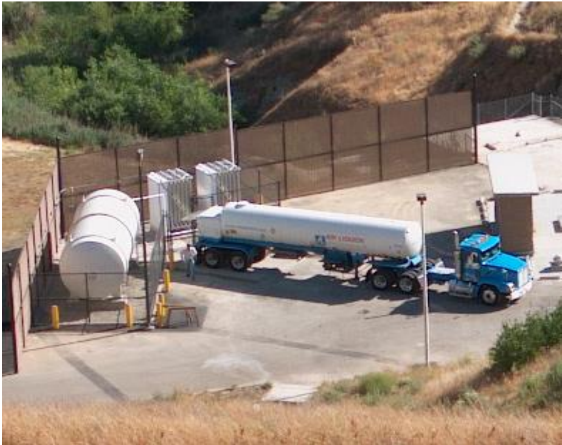
Figure 3-2: Example horizontal liquid oxygen tank, vaporizers, and delivery truck (Lake Casitas, Mobley Engineering)
