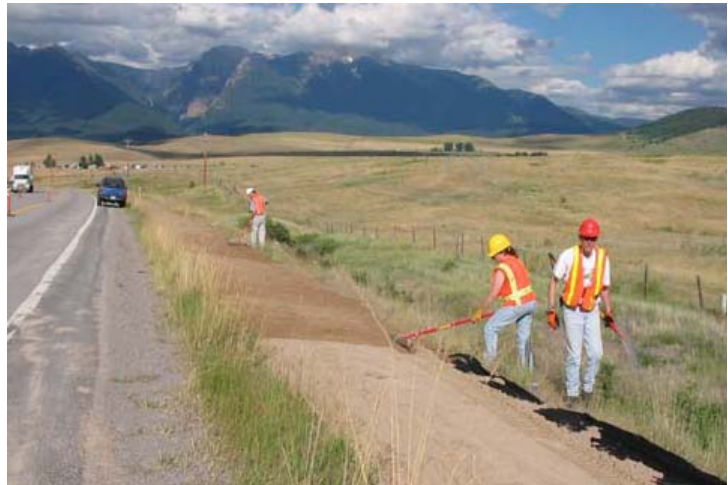
Figure 11: Installation of raked soil beds adjacent to US-93 in Montana (Montana DOT, 2006).
