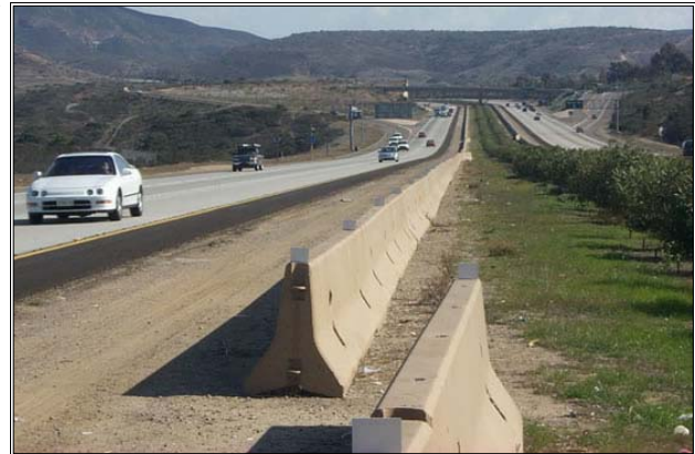
Figure 26: Median Barrier with gap. Caltrans photo.
