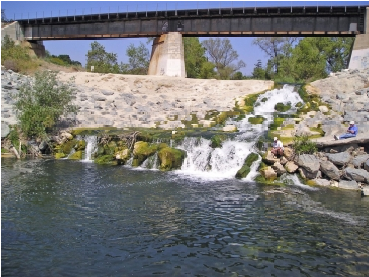
Metrolink barrier on Arroyo Trabuco Creek, tributary to San Juan Creek – 2009 Courtesy of Valerie Taylor, CDFW 4
